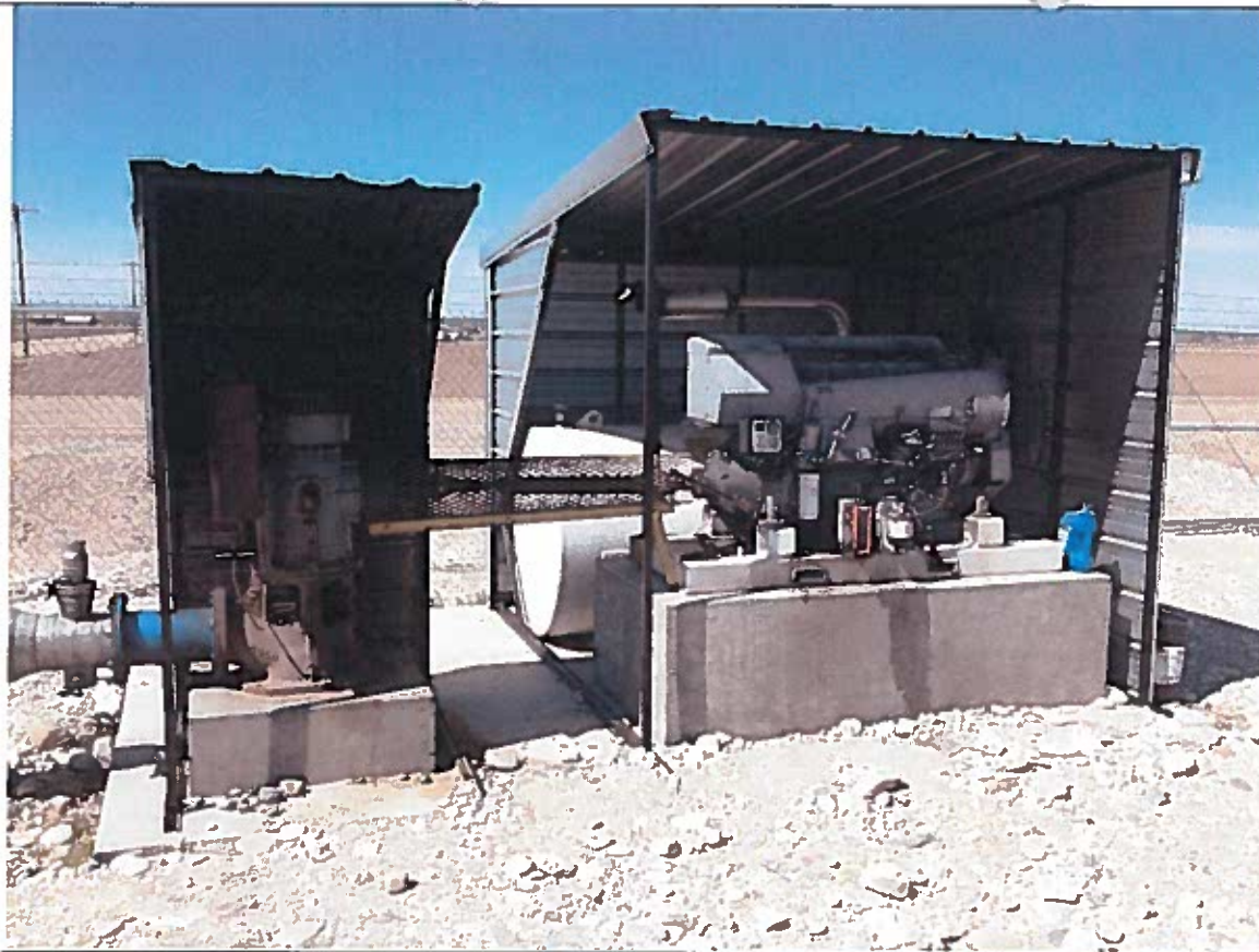
Well, pump and diesel motor.
