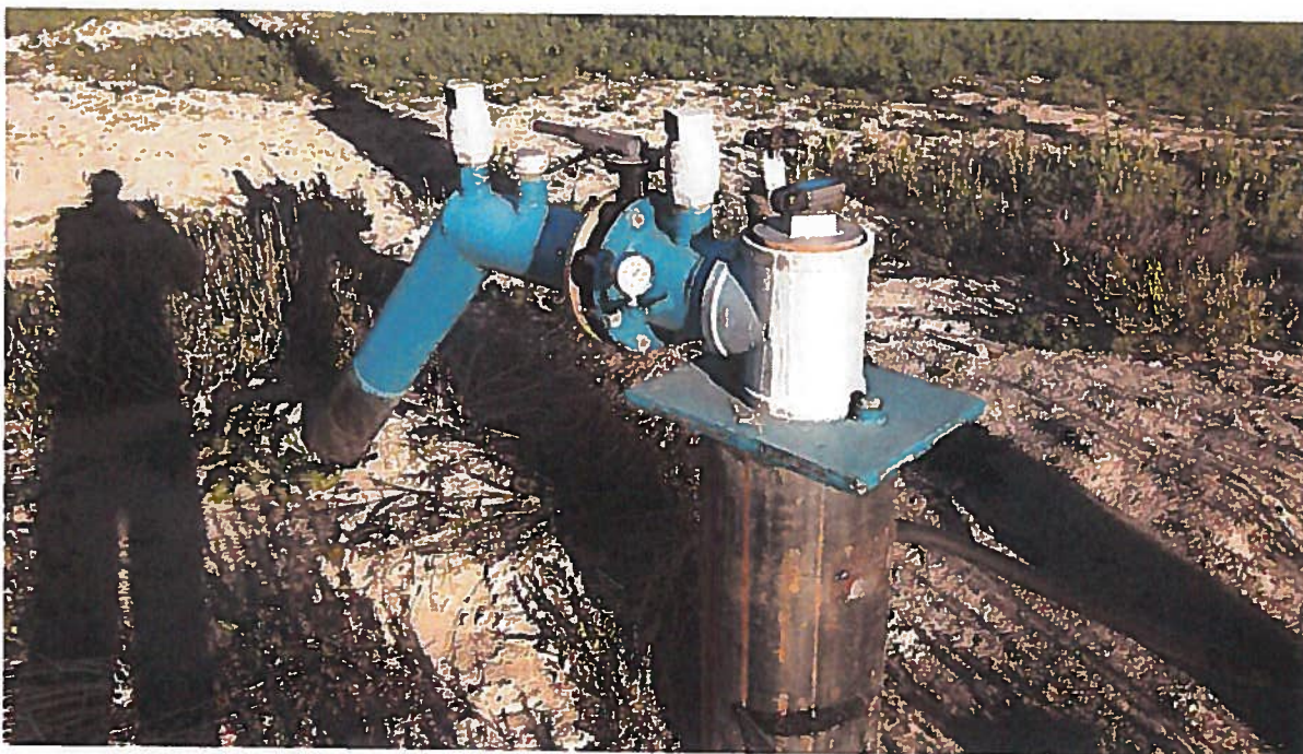
Photo 2. View of POD with pressure gauge.
