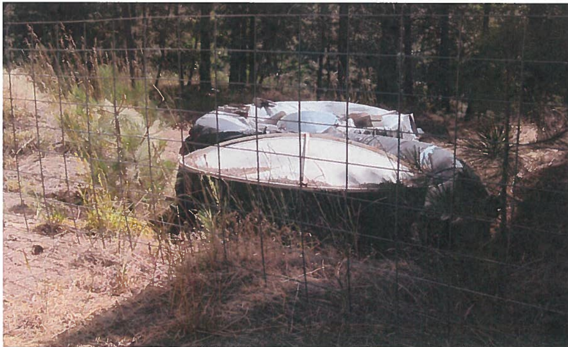
Fire protection - Water is pumped from Robie Creek to these two 600-gallon storage tanks.
