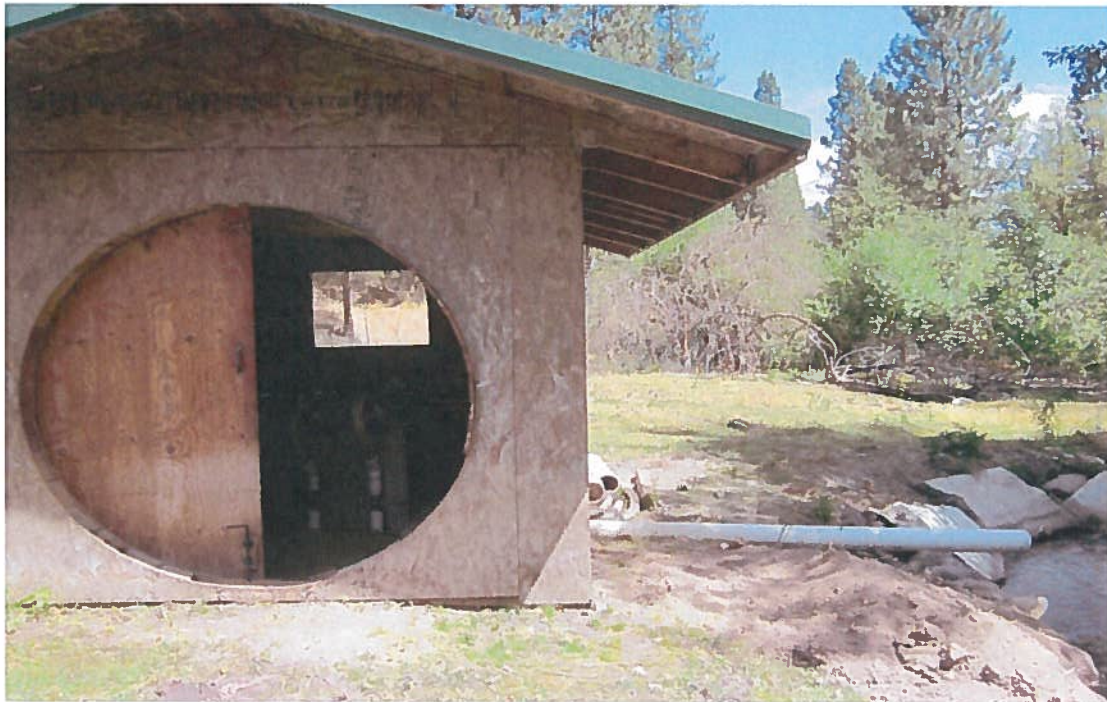
Power system – powerhouse. Discharge pipe to Robie Creek seen Right of powerhouse.
