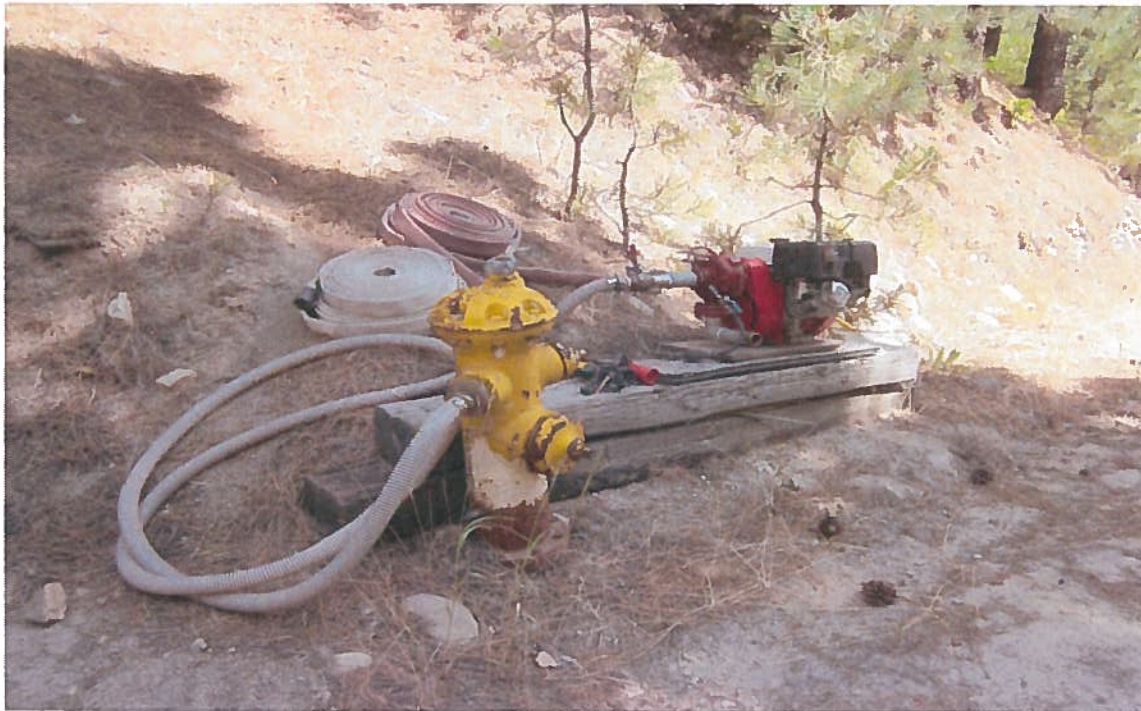
Fire protection system – water is pumped from the storage tanks to the hydrant as needed.
