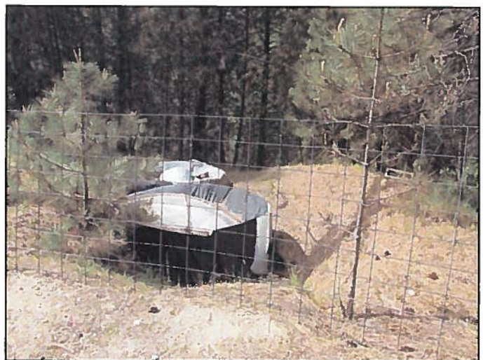
Fire Protection Tanks
