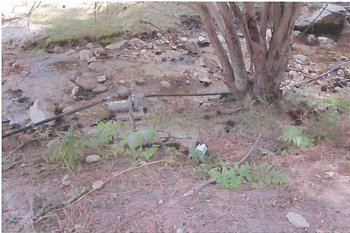
½ hp electric pump in Robie Creek for fire protection.
