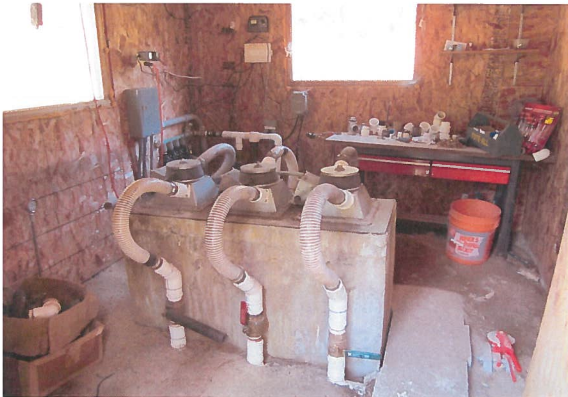
The 3 water turbines in the powerhouse. The 6" hoses that feed water to the turbines.
