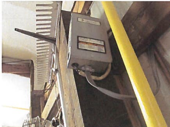
Control box for irrigation pump in barn
