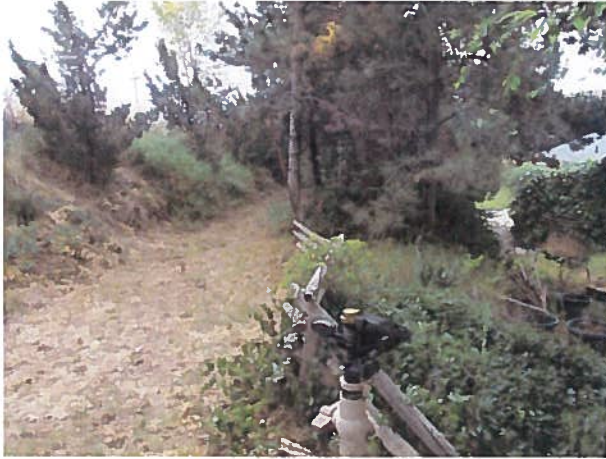
Sprinklers on risers beyond tree lines to irrigate landscaping
