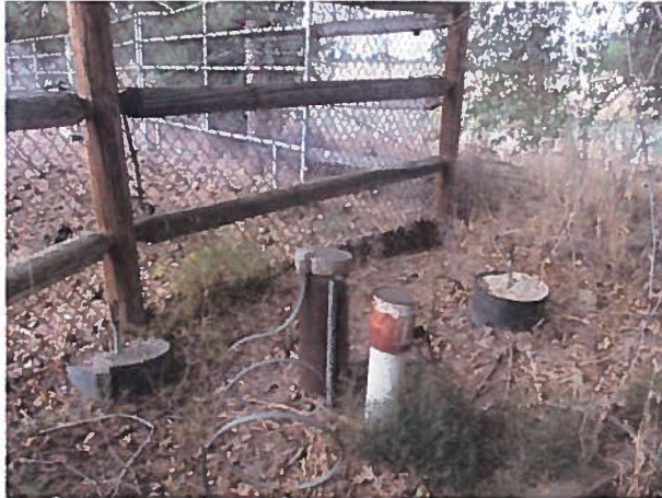
Well head for irrigation system (A0019181)
