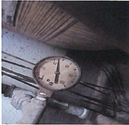
Irrigation pressure system
