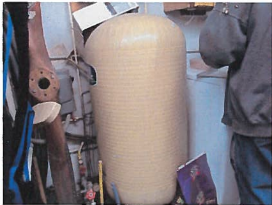
Pressure tank for irrigation system
