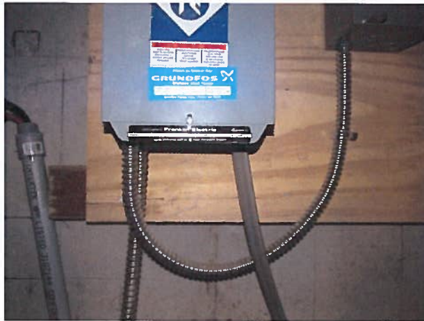
Control panel in room off of garage 5 hp pump
