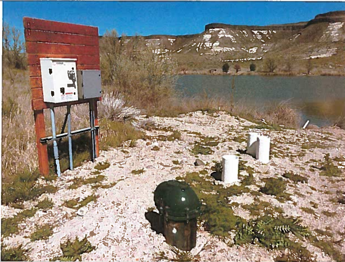
Well (D066241) is located south of the pond. Valves from Snake River and waste water direct flow into pond.
