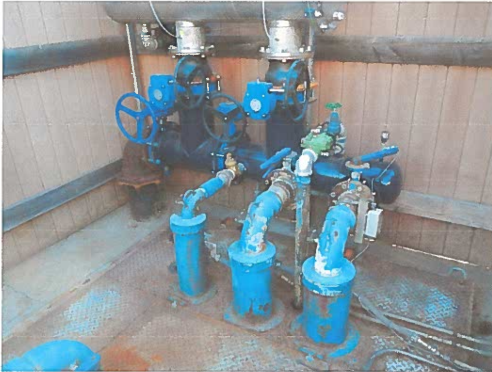
Manifold for Irrigation Pumps with Filter
