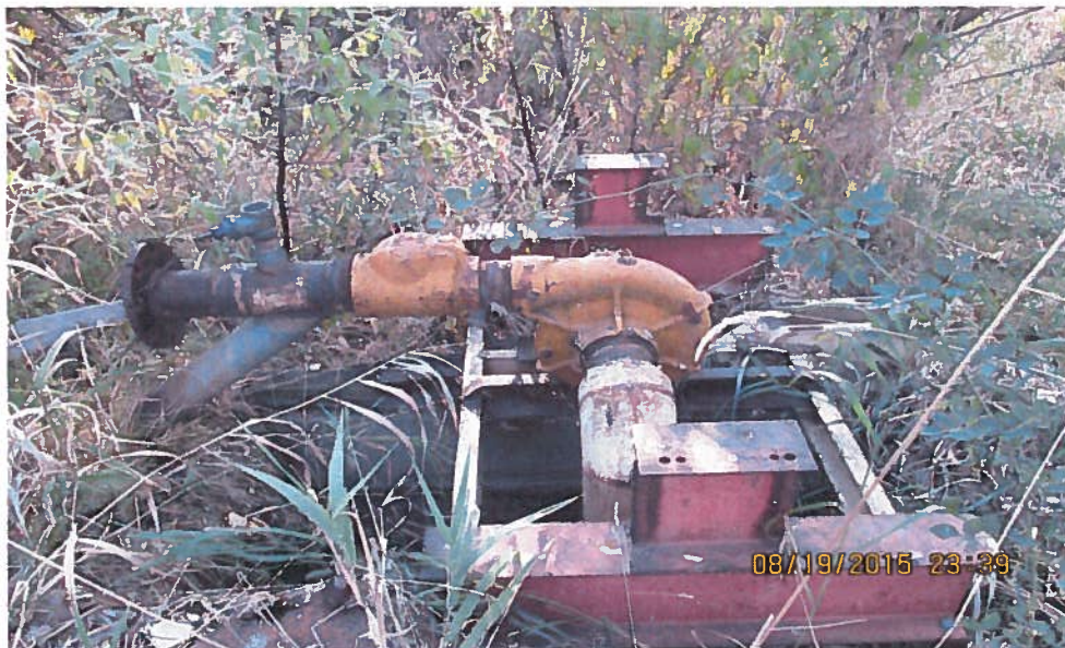
Pump for dry unnamed stream (wastewater source is only available for short period at end of irrigation season)
