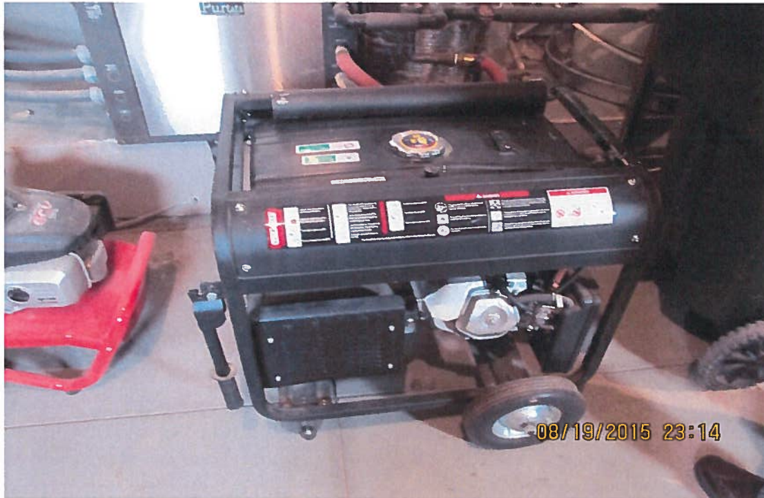
16 HP generator for running surface water pump
