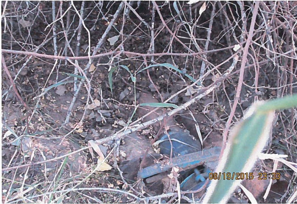
Control valve in dry unnamed stream
