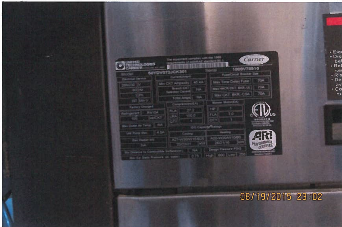
Heat exchange unit in garage
