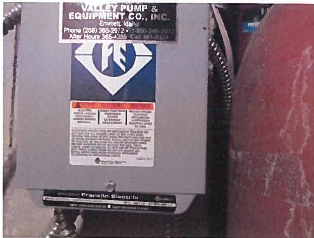
Pump Control Box
