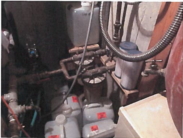
1" water line down to 2ea ¾" lines
