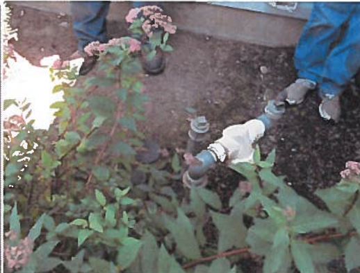
Filter for irrigation system old hook-up for Backflow taken from well-head
