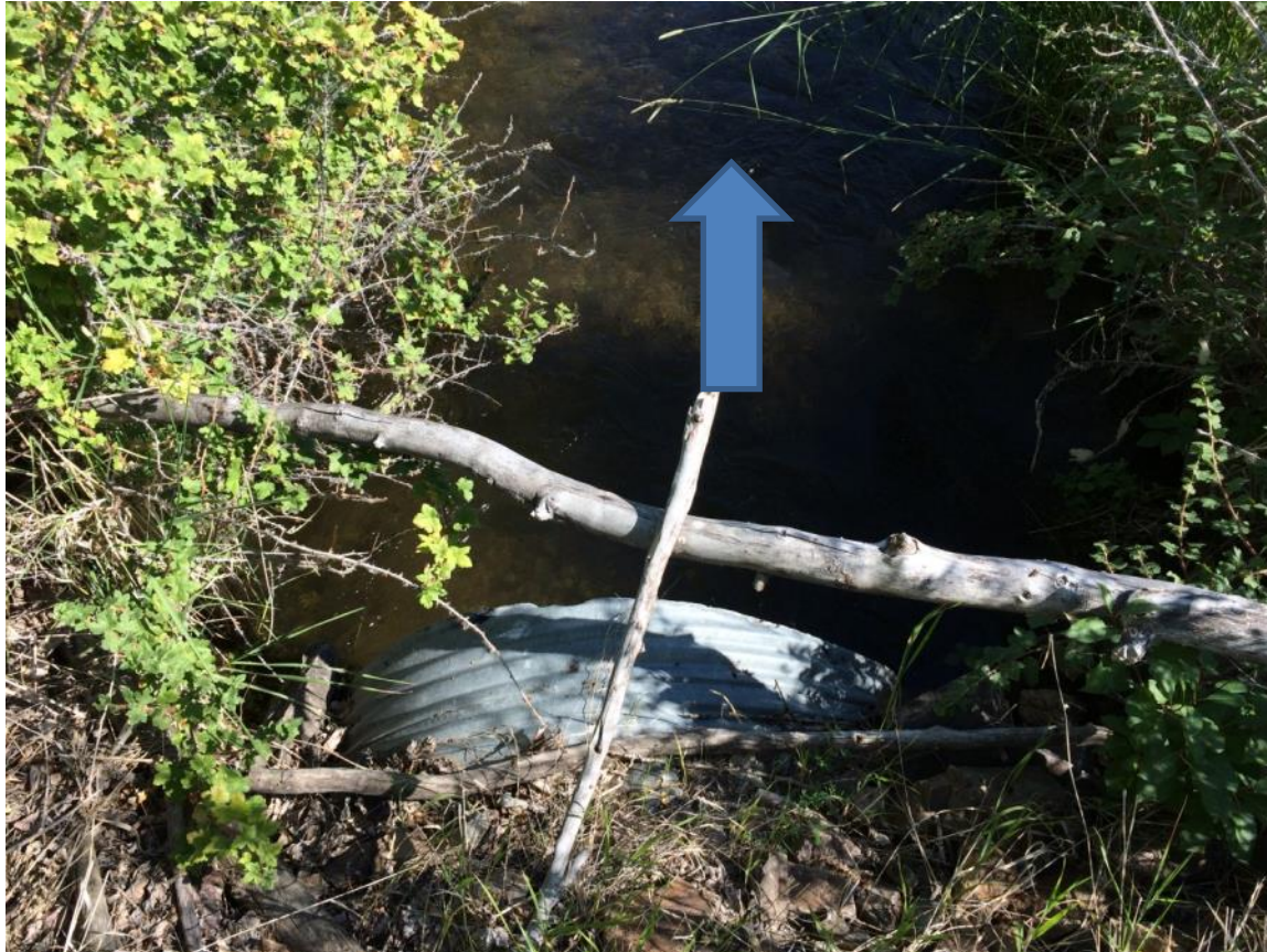
Culvert under berm with water flowing toward fish screen.
