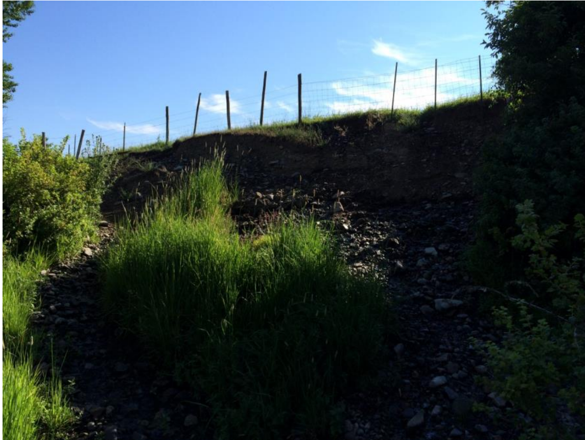
Seepage Springs/Wastewater near Check Dam
