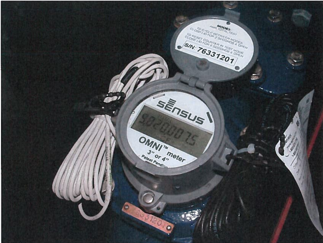
Well 5 - Flow meter
