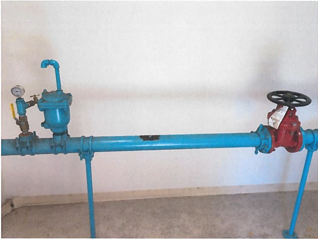
JD Well - Pressure gage, air valve, and isolation valve
