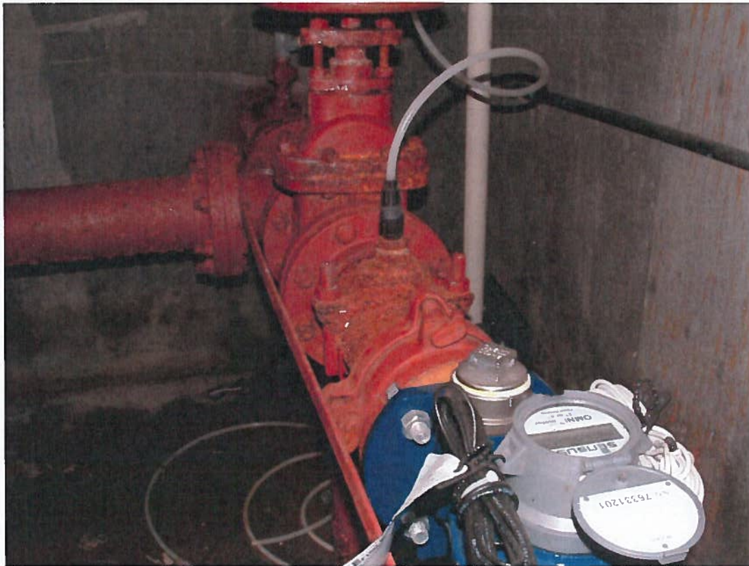
Well 5 – Piping exiting vault to system in background; to pressure relief and waste on left; chlorine injection in center
