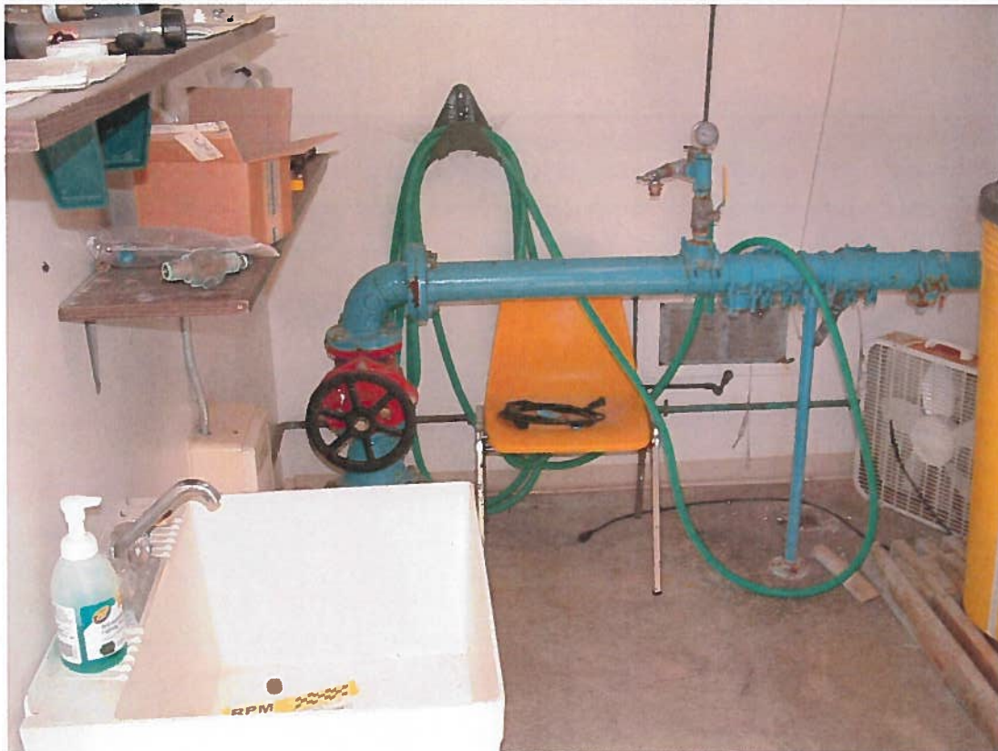
JD Well - Chlorine room; piping and pressure gage (90 psi)
