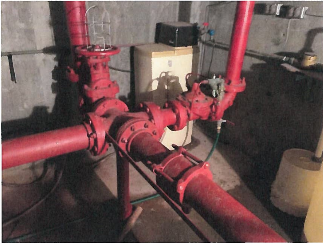
Well 5 – Piping; pressure relief on right, flush to waste in center background; chlorination system on right
