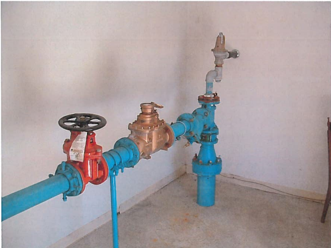
JD Well -Piping entering building, with check valve, pressure relief valve, flow meter, and isolation valve
