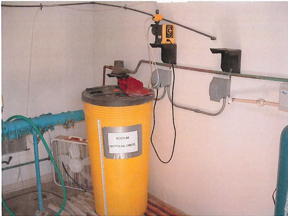
JD Well - Chlorine room; tank and chemical feed pump
