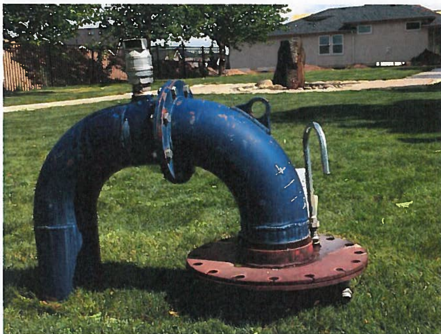
Figure 1. Supply well and submersible pump, looking approx. south
