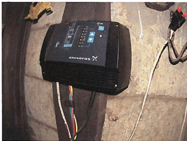
Domestic well controls
