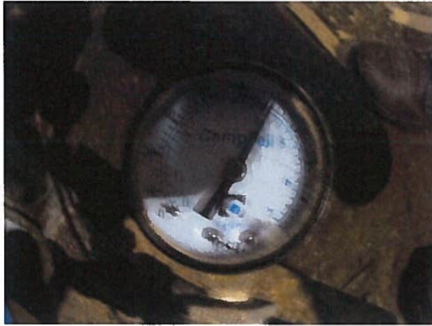
House pump is ¾ HP Pump set at 60 feet`
