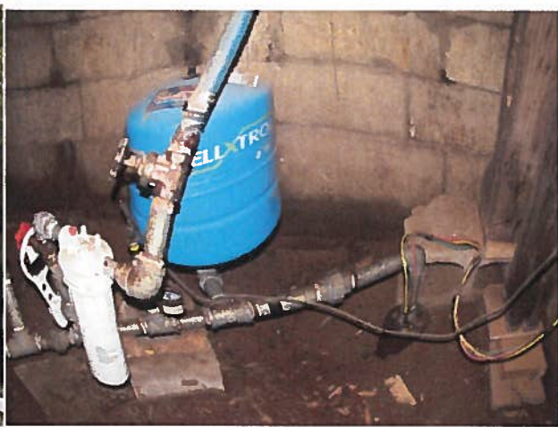
Domestic well inside shed
