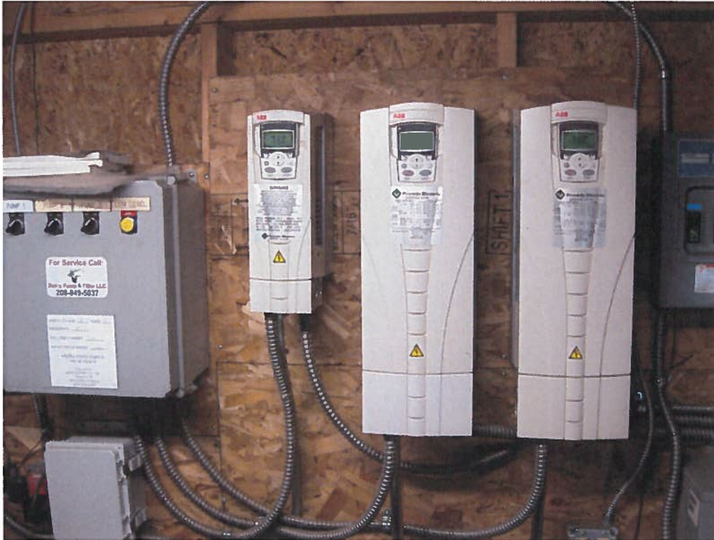
Three pump control boxes in the irrigation pump house.
