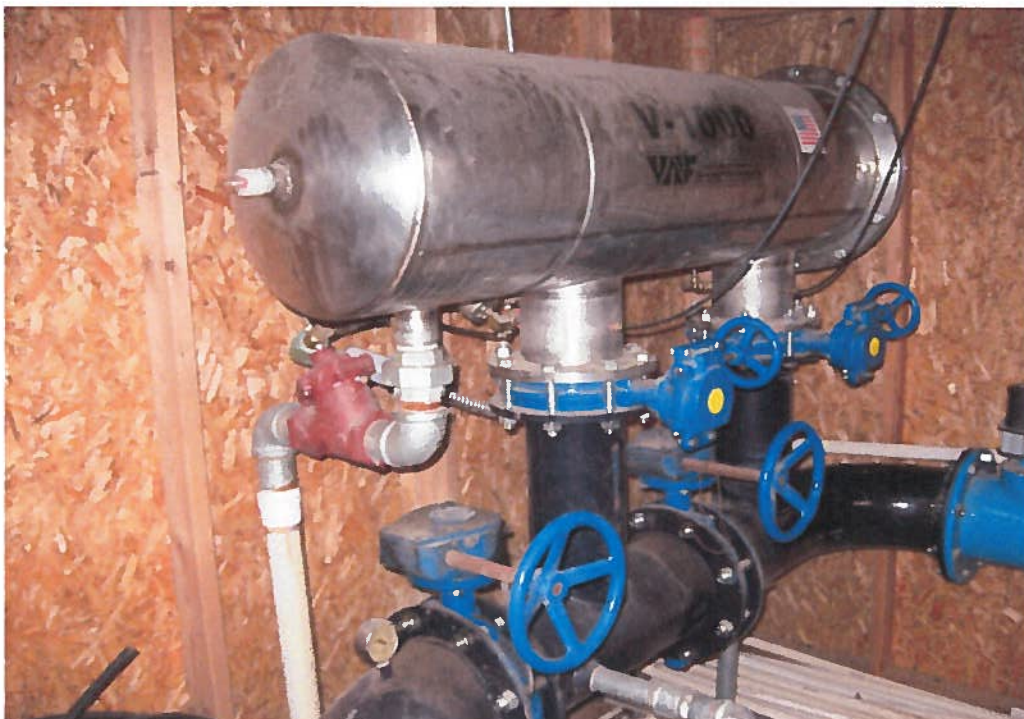
Inside of the irrigation pump house
