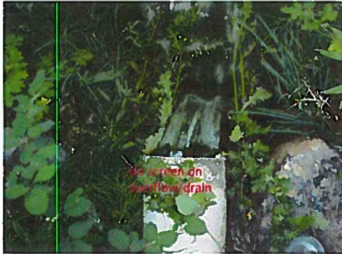
Photo 5. Overflow and drain for tank #1 –
