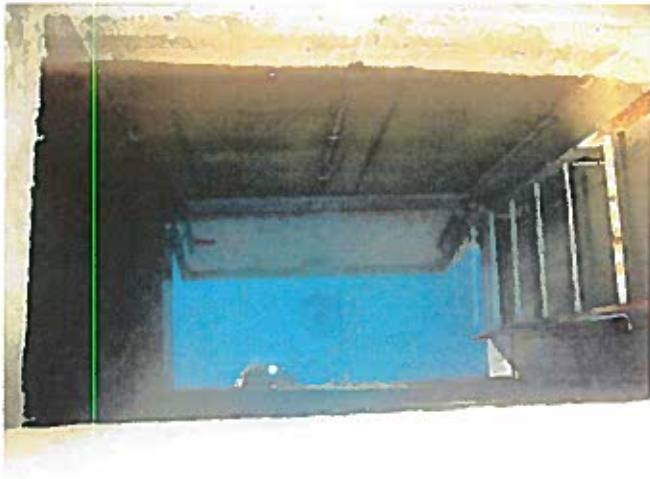
Photo 7. Tank #2 interior, no overflow.
