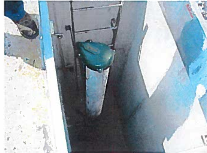
Photo 10. Well is raised above ground surface within the well vault.
