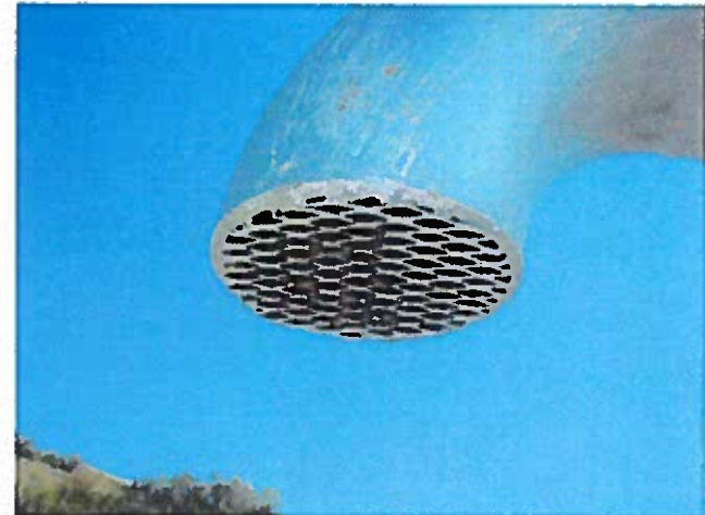
Photo 8. Tank vent for tank #2.
