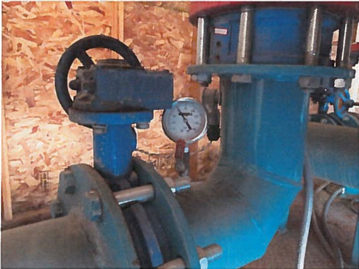
In line system pressure at 62 psi
