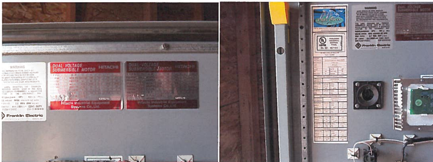
Well control panel
