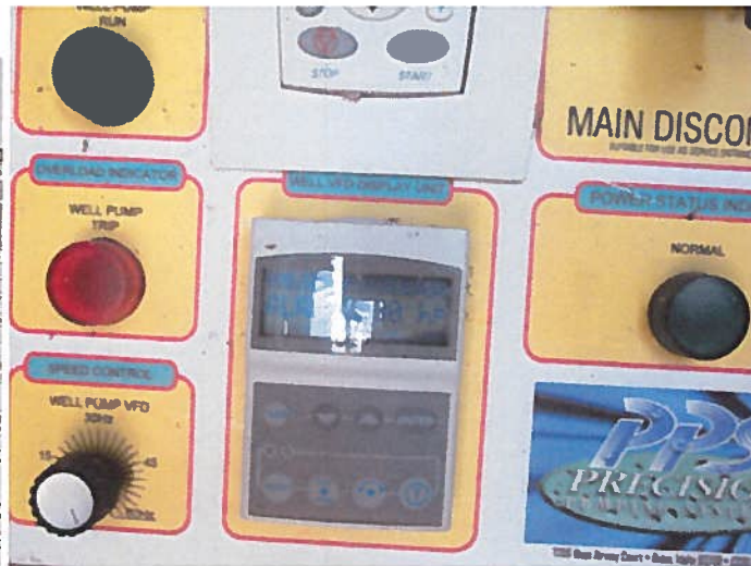
Control panel with well pump running
