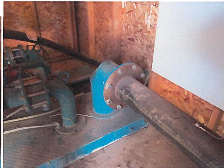
Pipe from well to vault and piping from vault to system
