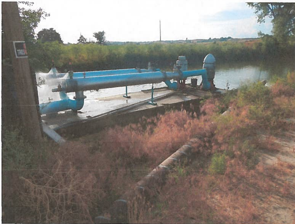
Rediversion pumps. Discharge from wells #1 and #2 in right of photo.
