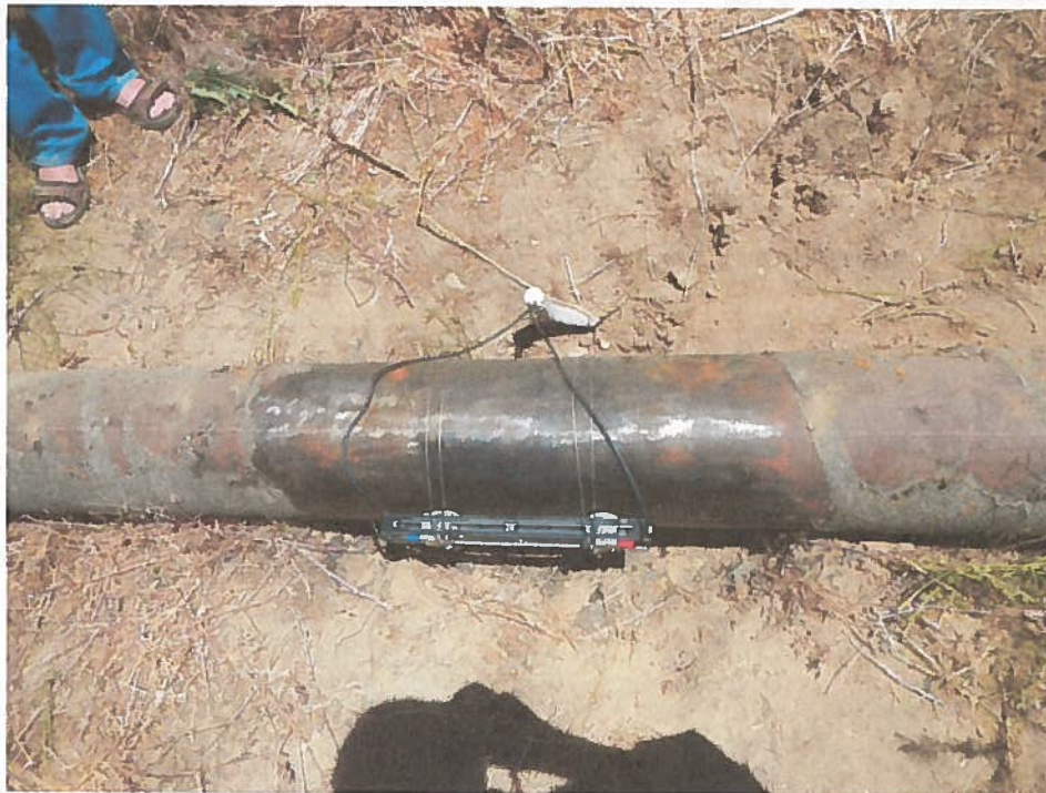
Transducer mounts for meter on old wells
