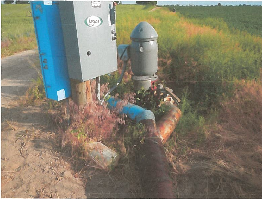
Well #1 foreground and pipe connection to well #2 discharge. Well #2 in background.
