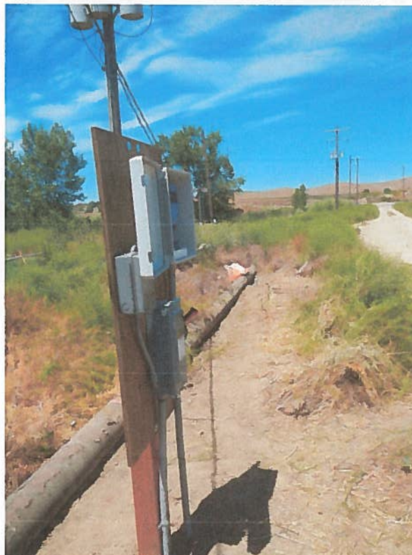
Meter readout in foreground and transducer location in background
