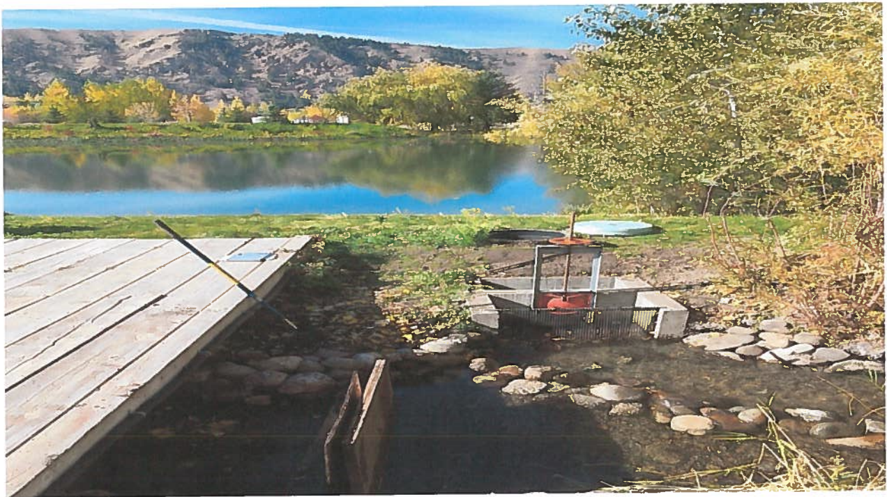
Inlet Structure and Flow Meter Enclosure
