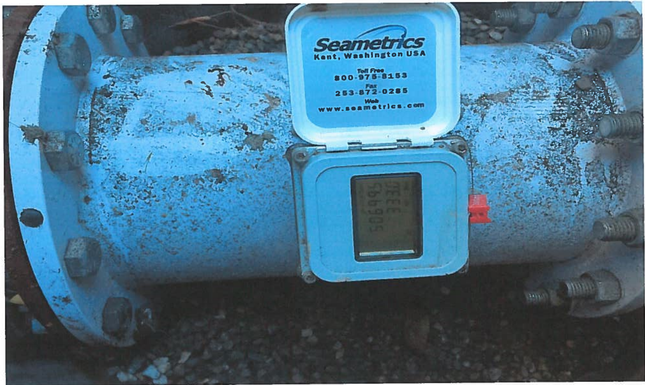
Inlet Pipe Flow Meter Note Discharge: 333 gpm
