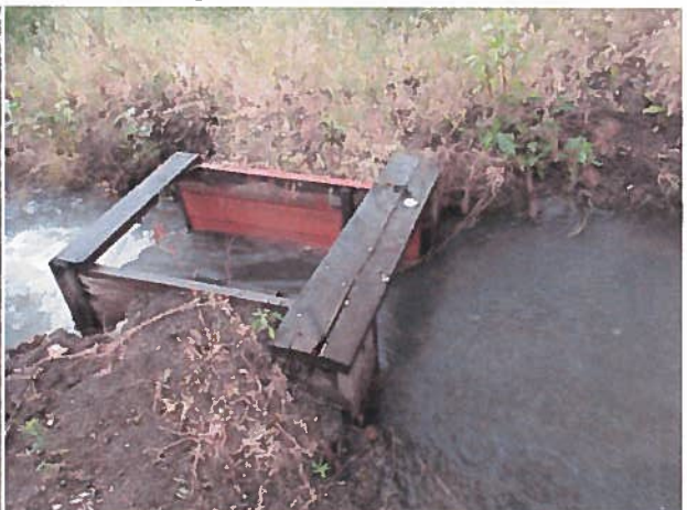
Irrigation control box for ditch
