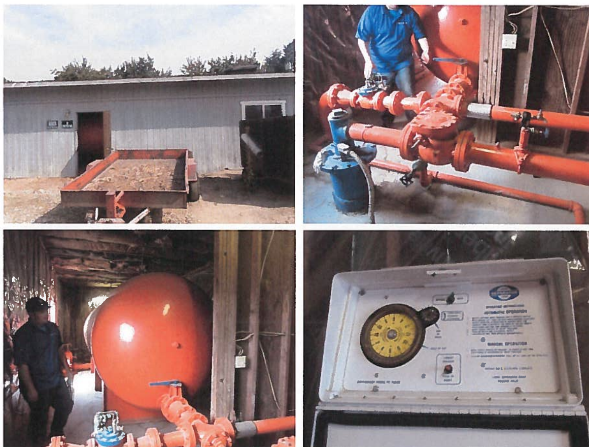
Well No. 3: The well house (upper left) is located separate parcel inside the Eagle Hills Golf Course storage yard. Jeff explained that this well (upper right) was taken offline in 1995 due to iron and bacterial contamination. A 4000 gallon storage tank (lower left) is also housed in the well house; it appears to have been connected to the system when the well was operational. The well house was dusty and cobwebbed, clearly indicating non-use. The separator/filtration system controller is pictured (lower right).
