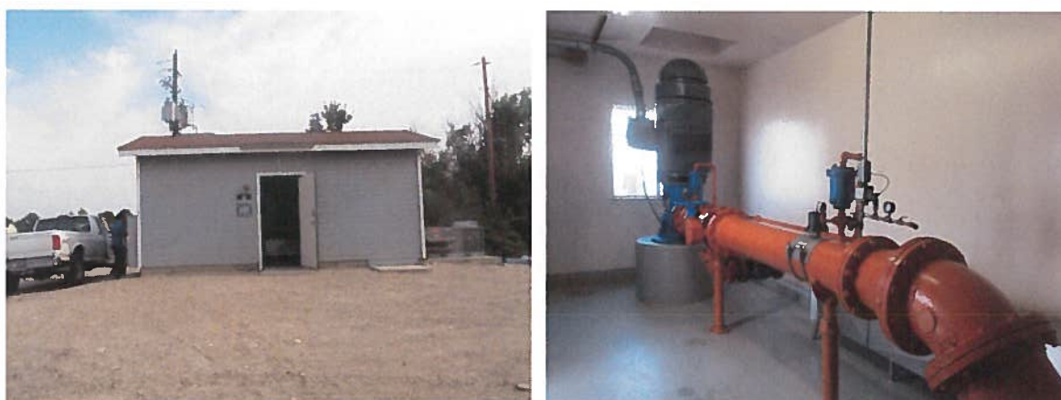
Well No. 4: It is located at the northeast corner of the Eagle Industrial Center campus at approximately 1800 E. State Street. Well No. 4 (300 hP) was on and pumping at the time of the exam; Layne brand pump was diverting approximately 1250 gpm (2.79 cfs).
