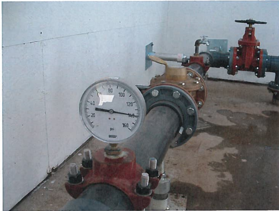
South well discharge piping (4-inch schedule 80 PVC). Check valve and flush to waste (out of picture in foreground), pressure gage, flow meter, sample tap, and gate valve for isolation.
