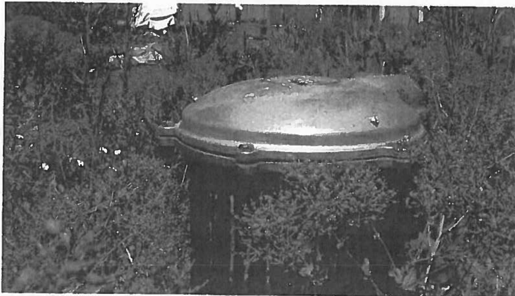
South Well casing and cap. Tag No. D0051999.
