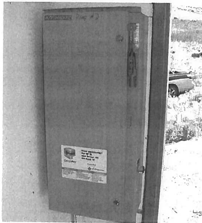
South Well pump panel. North Well panel is identical.
