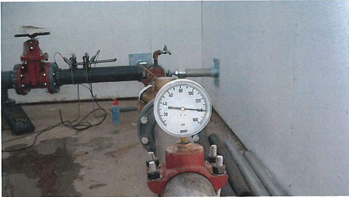
Calibration check of North Well flow meter. Installed Neptune meter behind pressure gage, portable ultrasonic flow meter on left.
