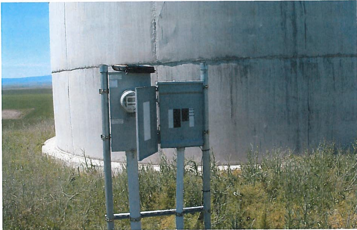
Circuit breakers for booster pumps (3-phase 100a, 20a, and 20a, and 1-phase 20a). Power meter #12578873 Clearwater Power Company. Electrical permit #6659981, 4/4/08 inspection date.
