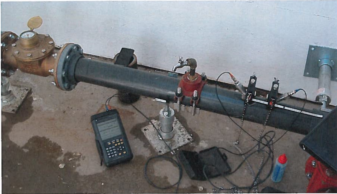
Calibration check of South Well flow meter. Installed Neptune meter on left, portable ultrasonic flow meter on right.
