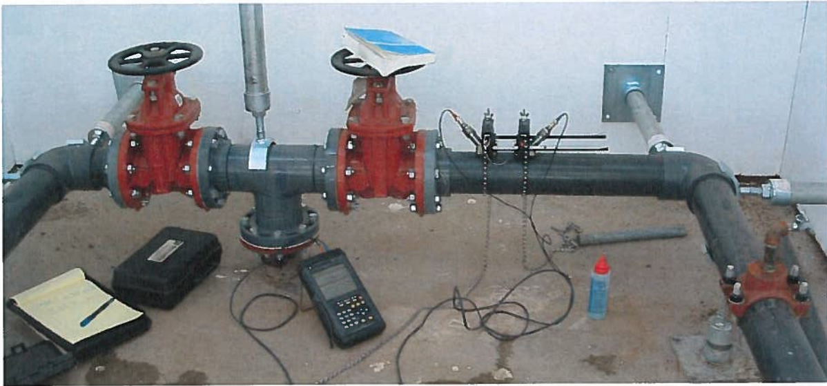
North and South Well piping connect between gate valves and discharge downward through floor to system
