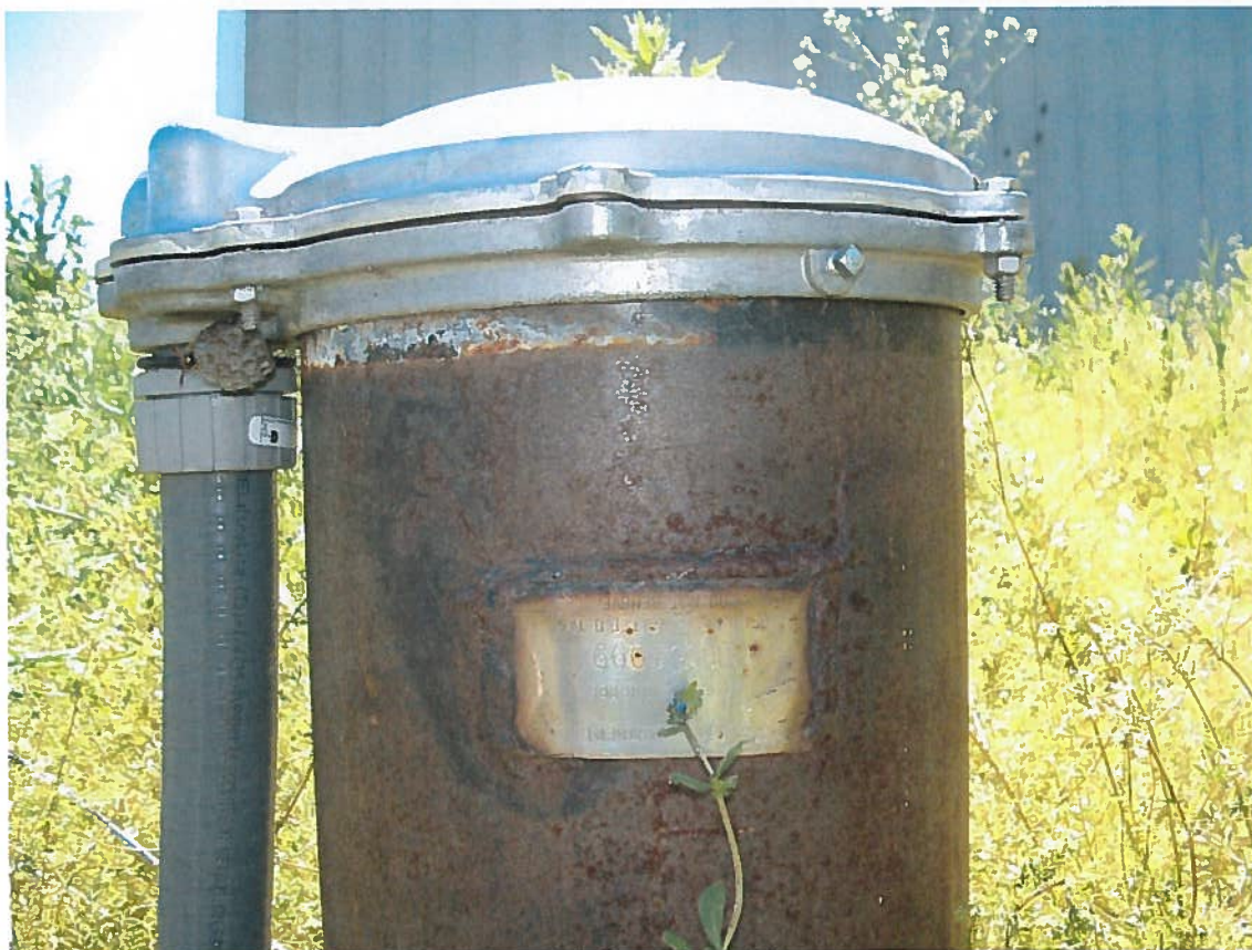
North Well casing and cap. Tag No. D0051998.
