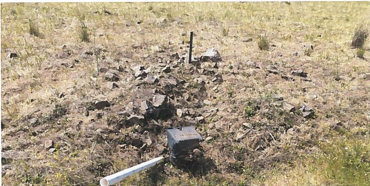
Blow-off valve at terminus of dead-end line extending south from well along Powell Road. Fence post in background is marker for buried stubbed pipe with curb stop (typical for each lot)
