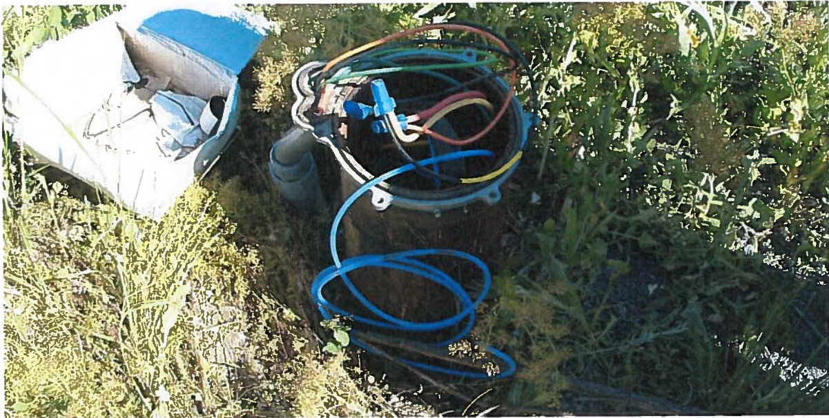
Inside North Well Casing. Blue tubing is air line for water level measurement.
