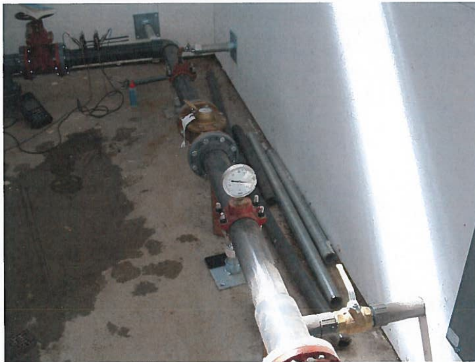
North Well discharge piping (4" PVC). Check valve (out of view in foreground), flush-to-waste pipe and ball valve, pressure gage, flow meter, sample tap, and gate valve for isolation.
