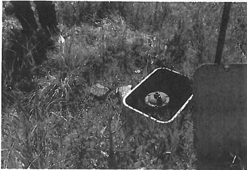
Air release valve at high point between wells and tank.
