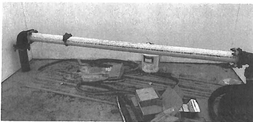
Interior of booster pump building. Piping is connected and pressurized through building, but waiting for booster pump installation to provide adequate pressure (>40 psi) for high elevation lots
