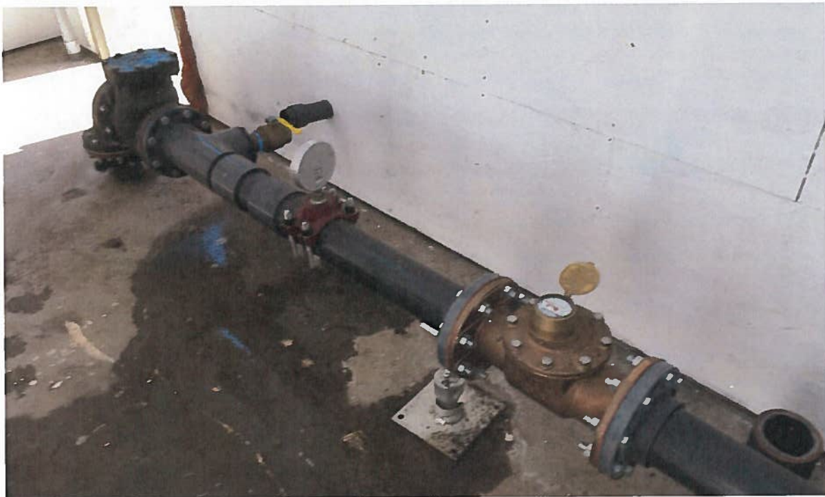
South Well discharge piping. Check valve on left, then flush-to-waste, pressure gage, and flow meter.
