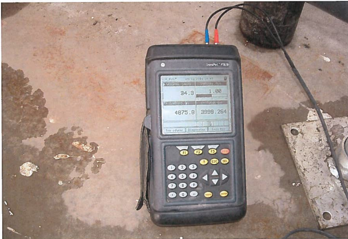
South Well flow rate is 34 gpm with ultrasonic meter and 33 gpm with Neptune turbine meter; 138 psi discharge pressure.
