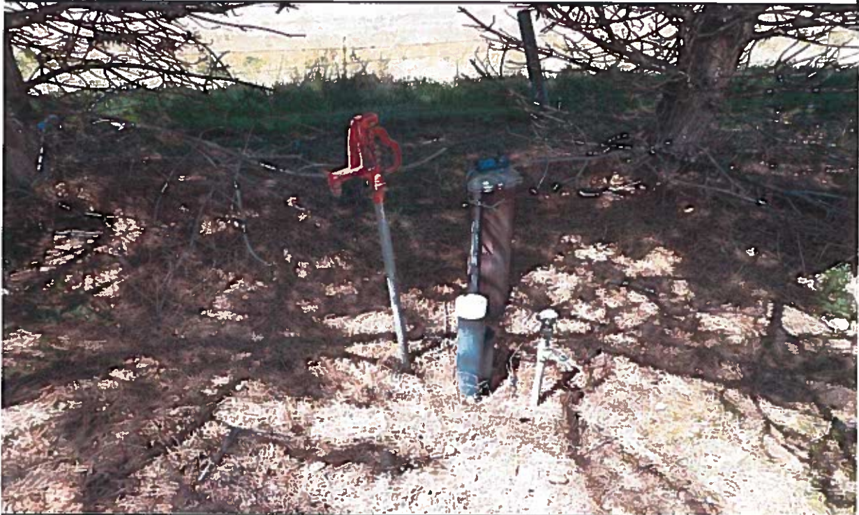
Point of Diversion: View northerly of the ground water irrigation well located in the northwest corner of the right holder's property.
