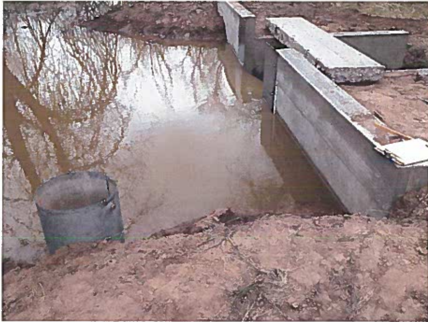
Figure 3: 5' Rectangular Weir with staff gauge on ditch
