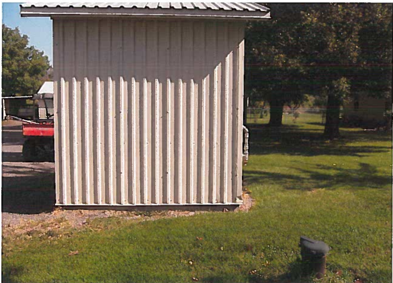
Below: Pump House and Well Head
