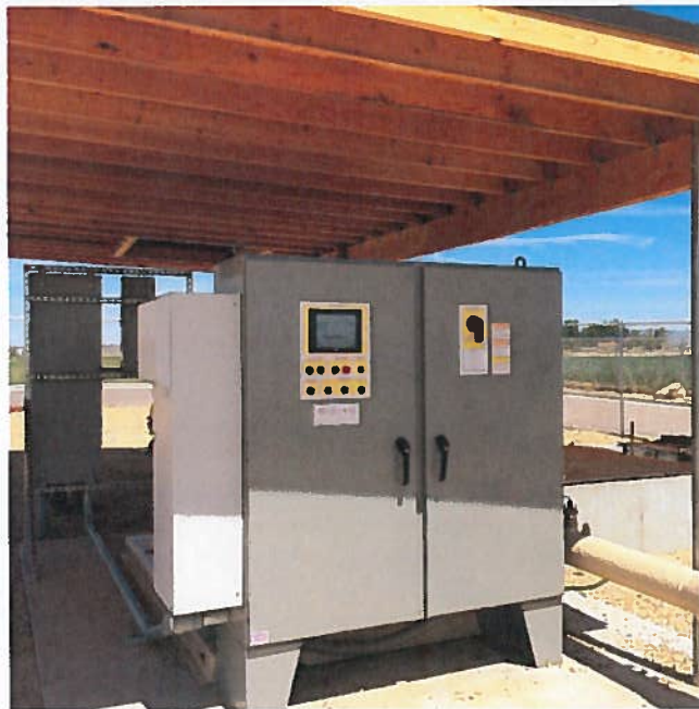
Figure 6. Control panel for surface and ground water, which are operated independently; looking north
