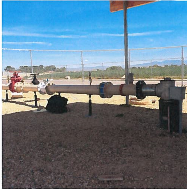
Figure 1. Well is equipped with 30 hp submersible pump, looking northeast
