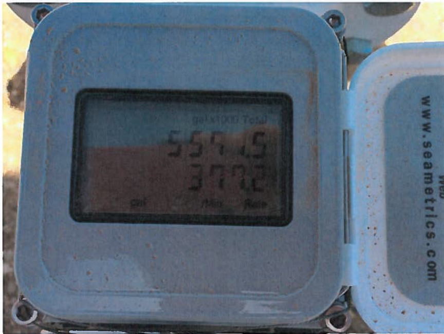
Figure 5. Magnetic flowmeter reading during testing
