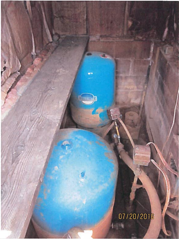
Pressure tanks, one for each well
