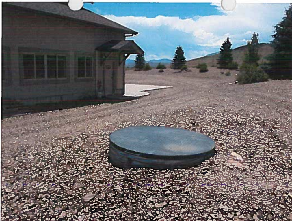
Point of diversion – well
