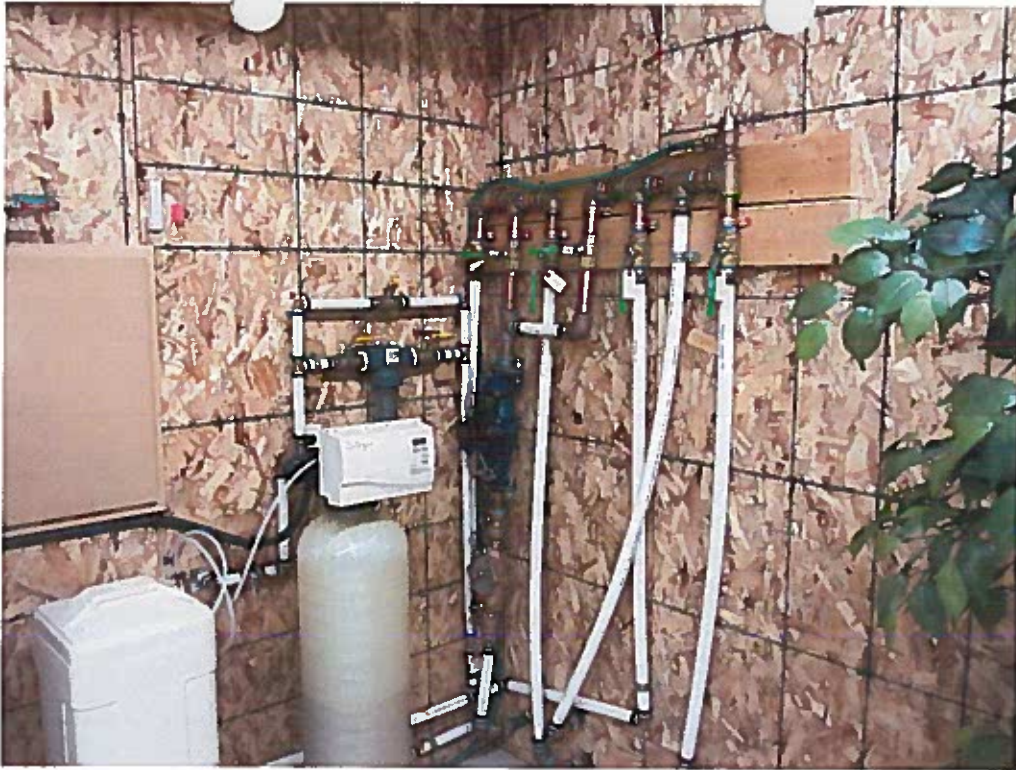
System plumbing in basement of Watson home
