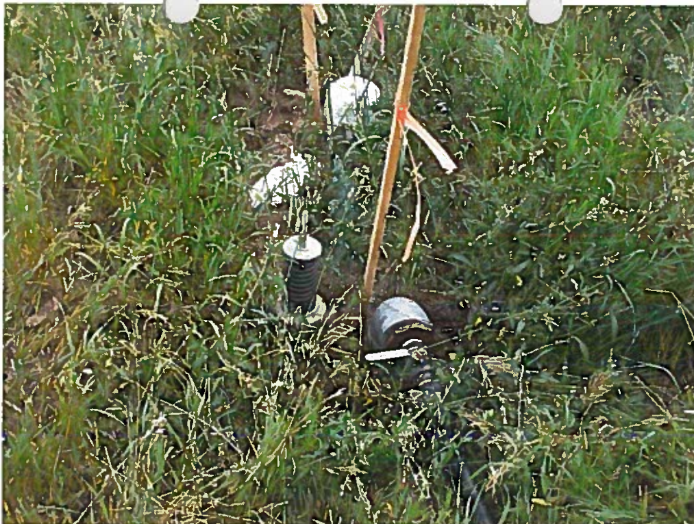
Riser and valve for irrigation system
