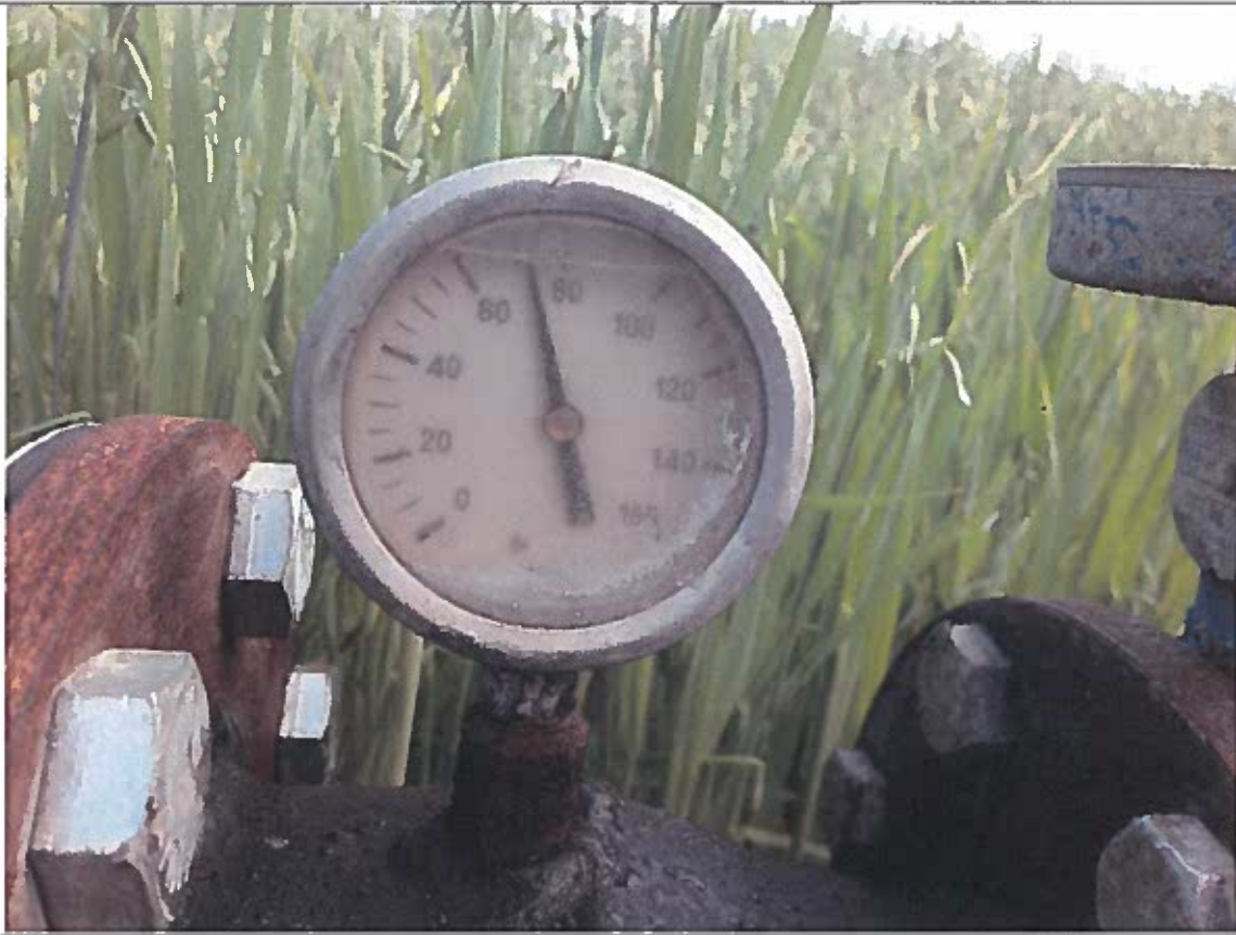
Pressure gauge on east well reads 72 psi.
