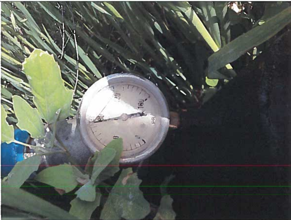
Pressure gauge on mainline reads ~75 psi.
