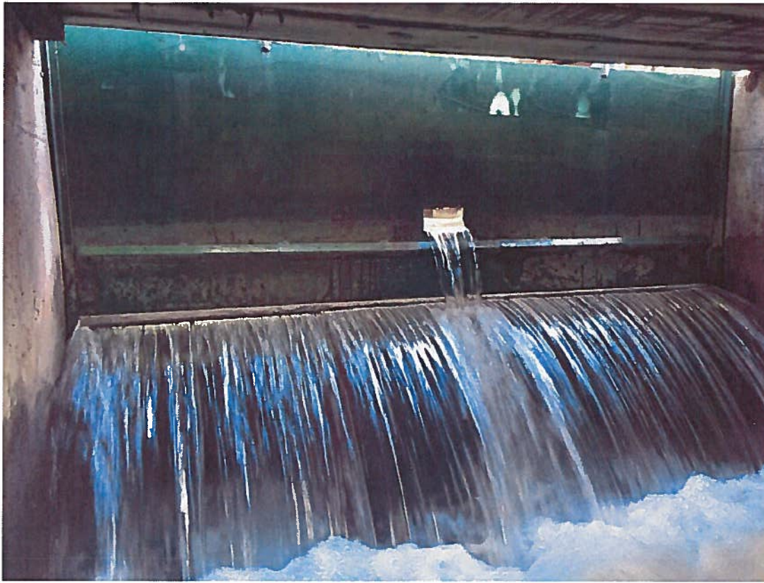
Figure 7: Downstream Side of 8' Vertical Slide Gate and Custom Sharp Crested Weir.
