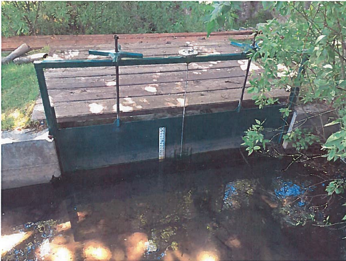
Figure 6: 8' Wide Vertical Slide Gate with Custom Opening and Staff Gauge.
