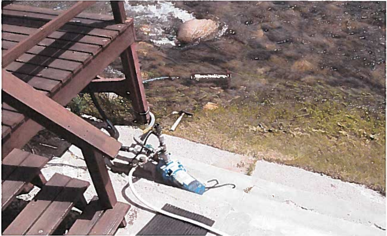
Above: Pump and Fish Screen from Salmon River
