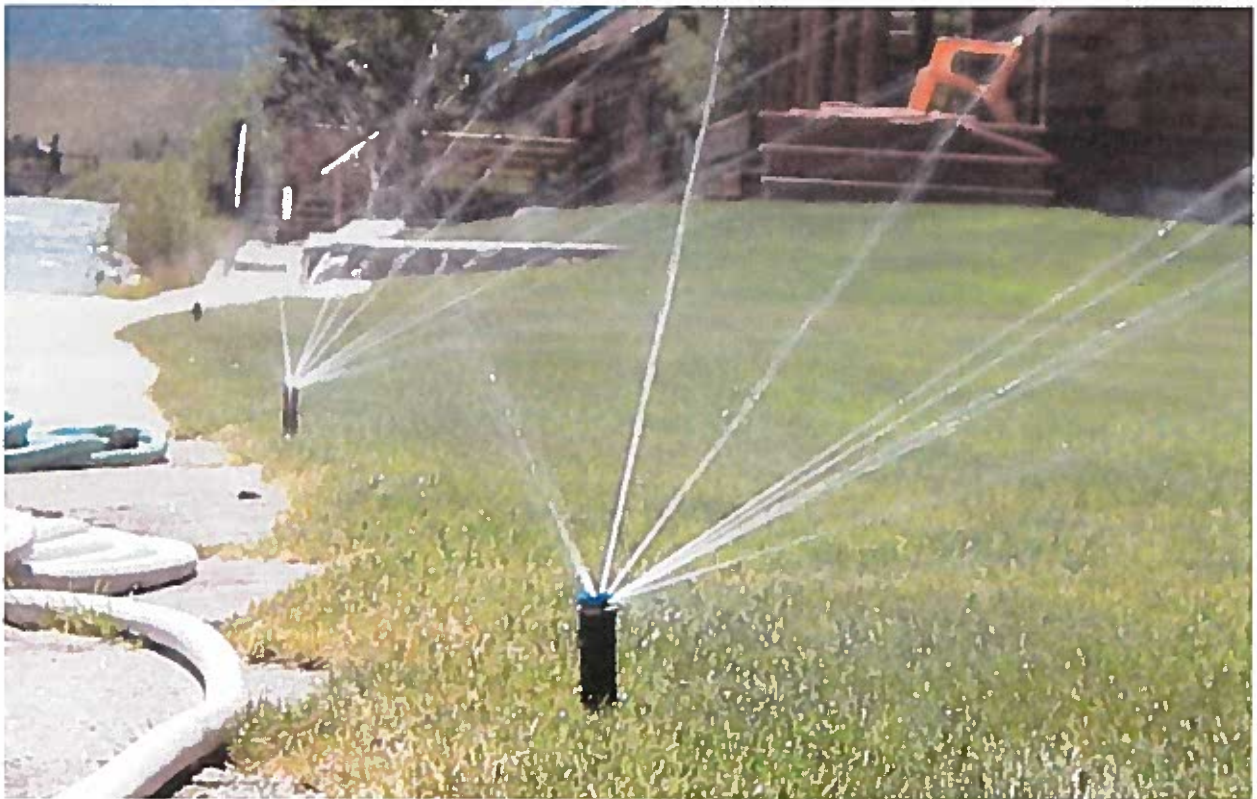
Above: Sprinkler System for Lawn
