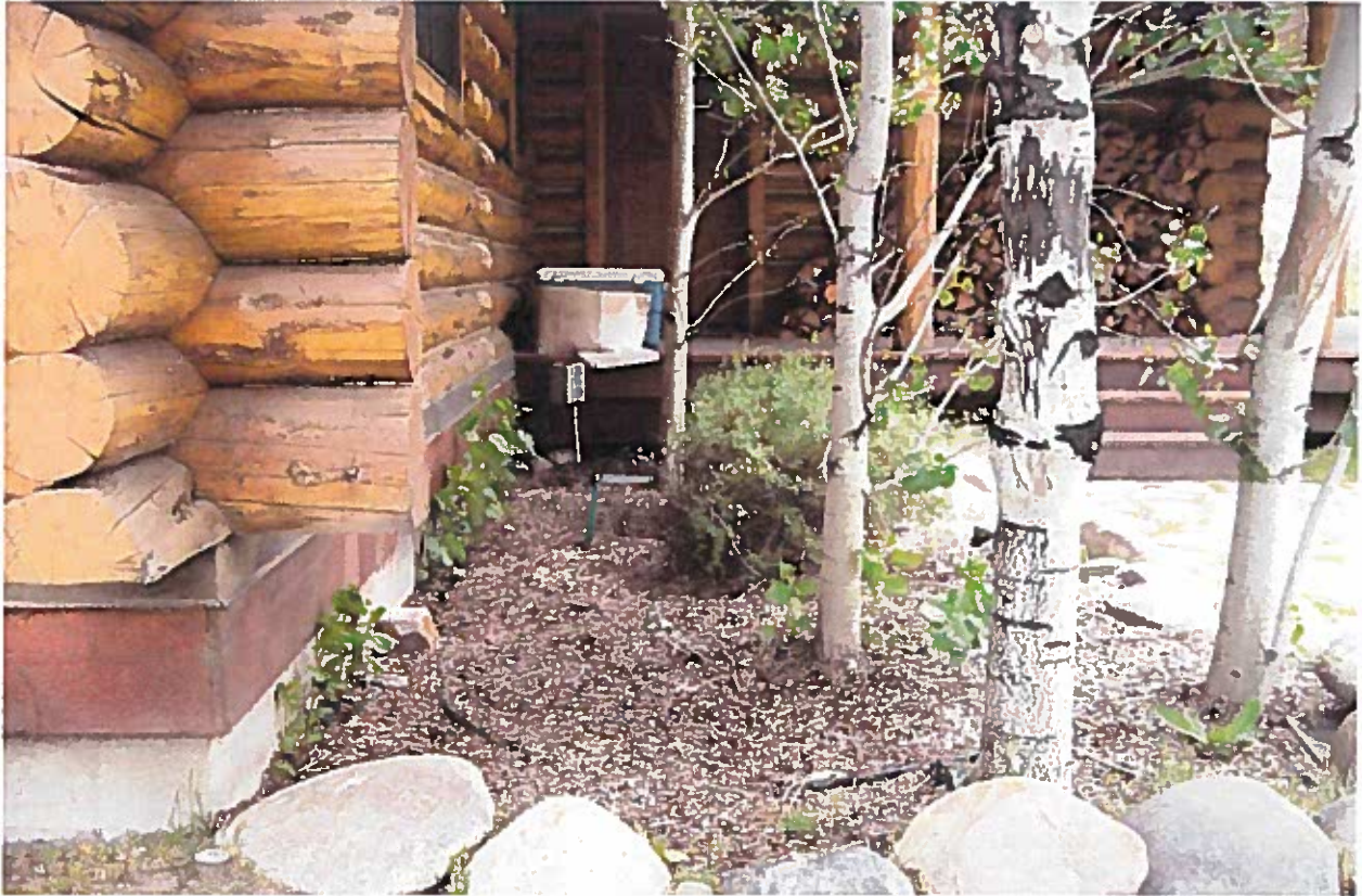
Above: Irrigation System Control Boxes
