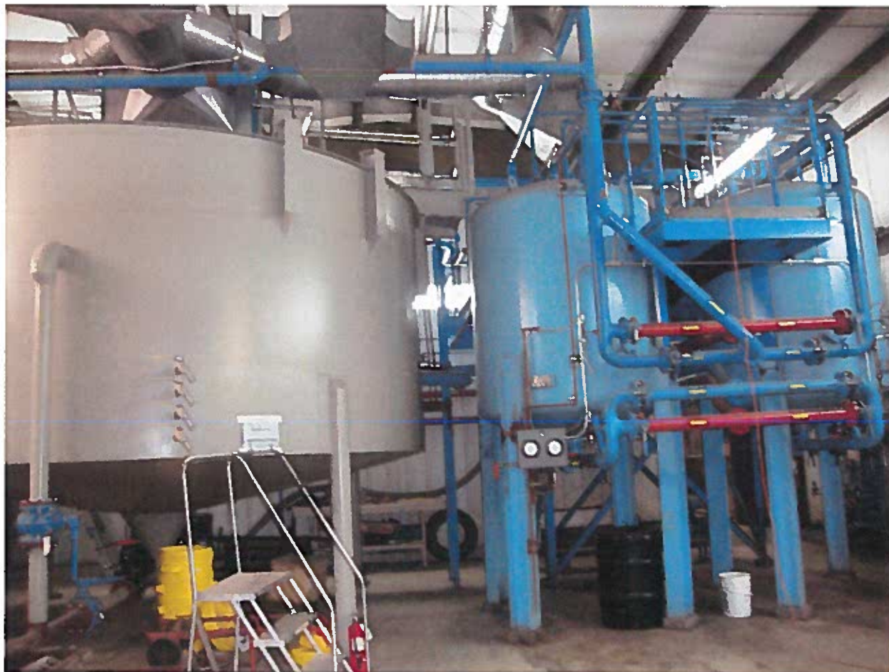
Below: Looking at the settling tank on the left and the carbon filters on the right.
