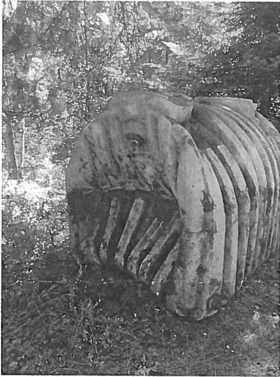
Photo showing snow damage to existing water tank which necessitated replacement
