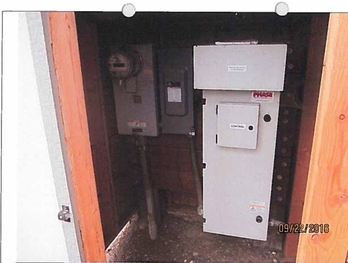
Inside the pump house
