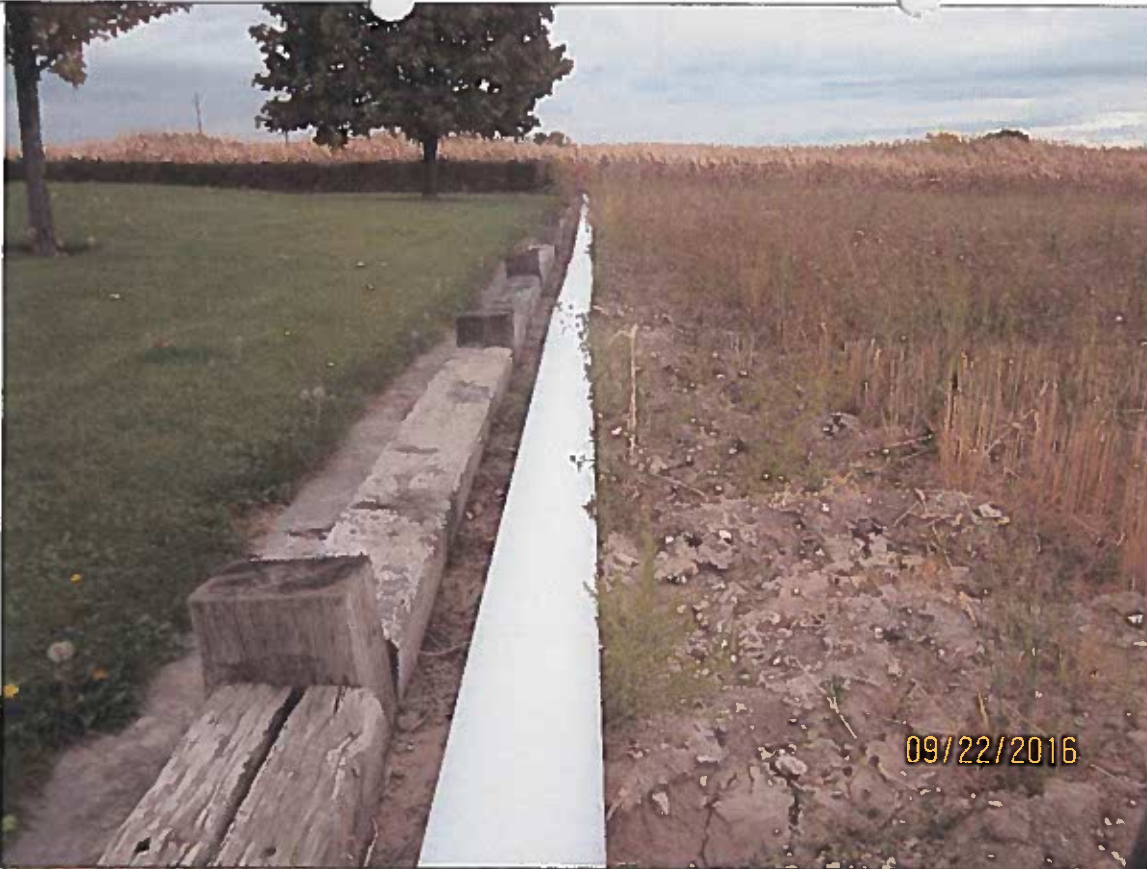
Above ground 8" PVC pipe for flood irrigation.
