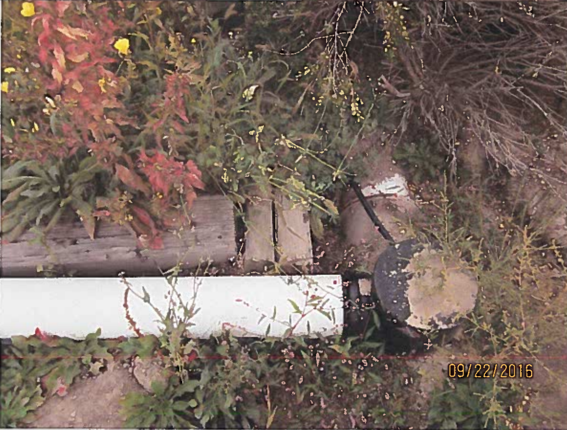
12" PVC reducing to 8" PVC. The 12" line runs along the bushes south of the house sitting on the west side of McDermott Road.
