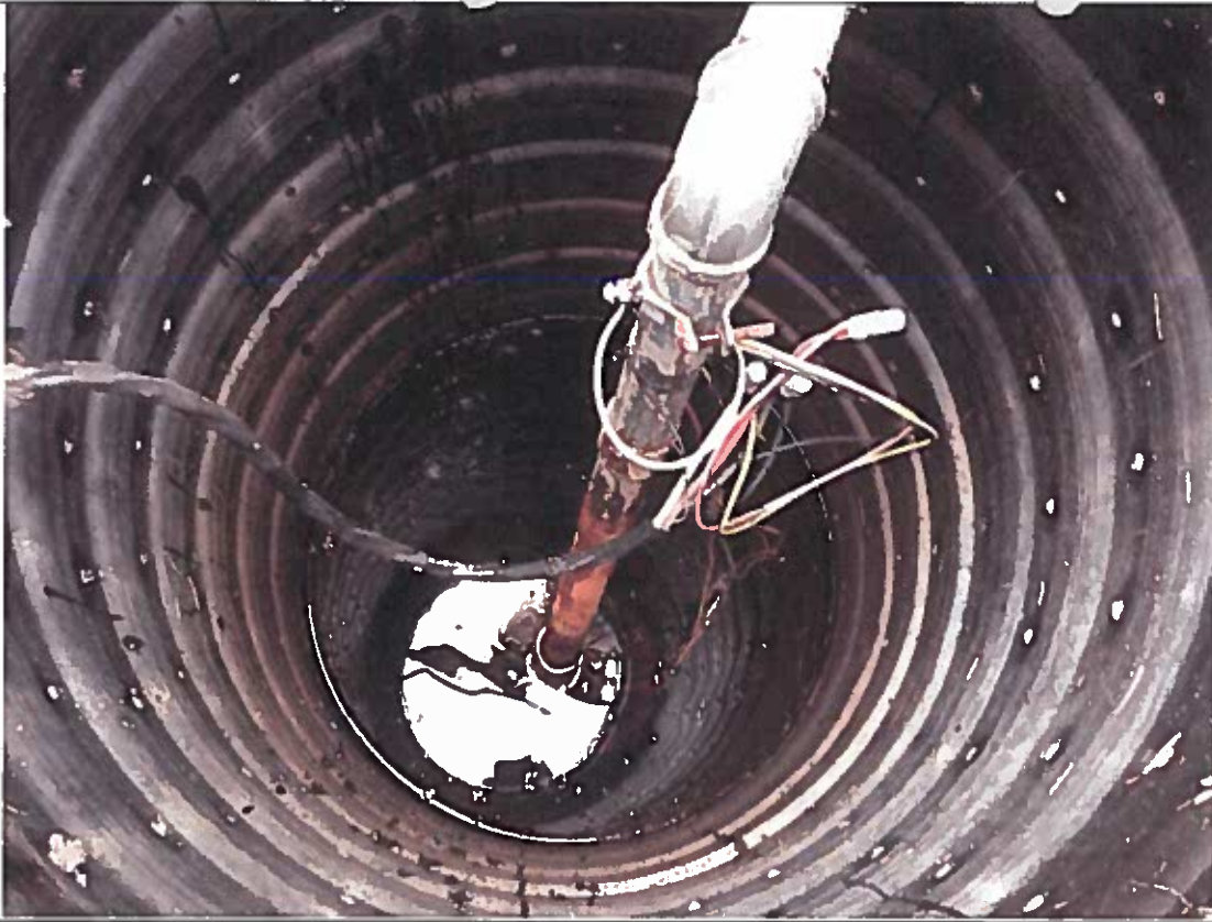
View of submersible 10hp pump
