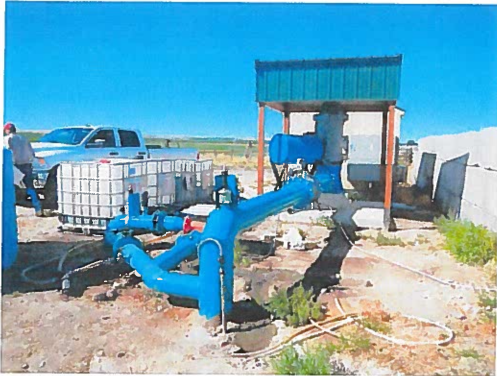
Photo 6 – Booster Pump Connection at New Well 2
