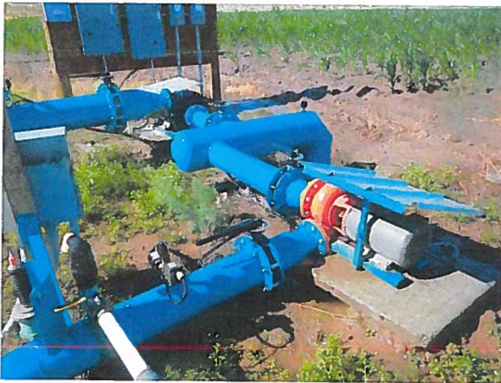
Photo 7 – Booster Pumps Located in Section 17
