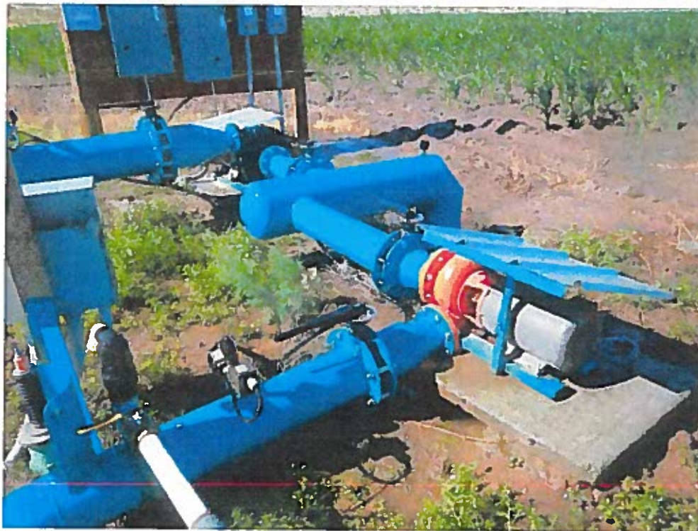
Photo 7 – Booster Pumps Located in Section 17
