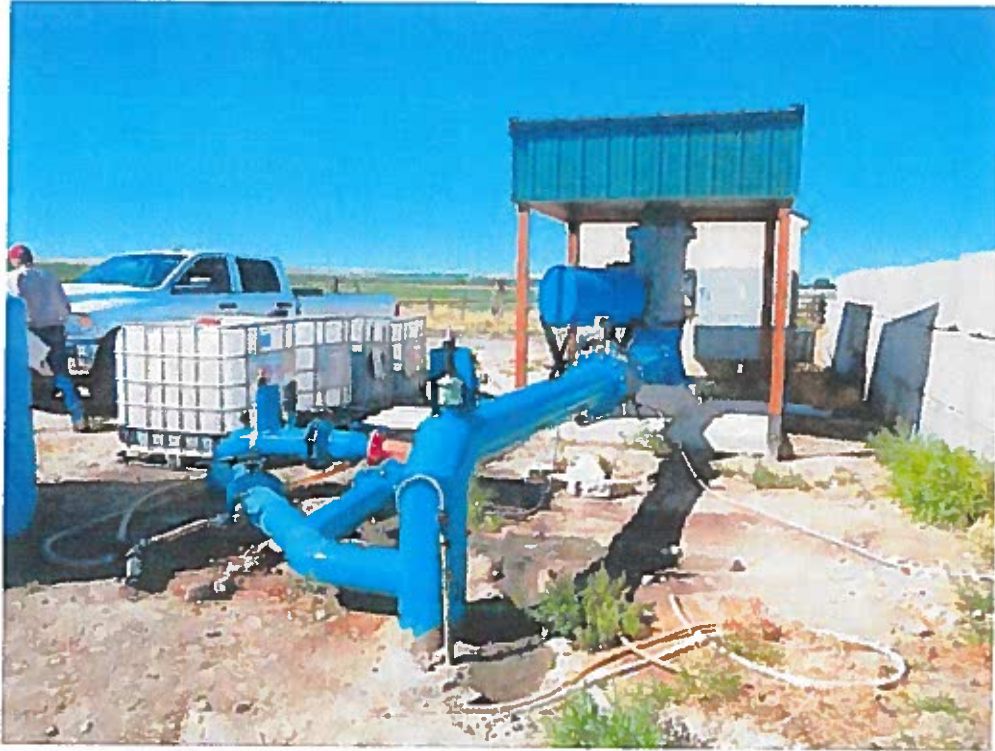
Photo 6 – Booster Pump Connection at New Well 2
