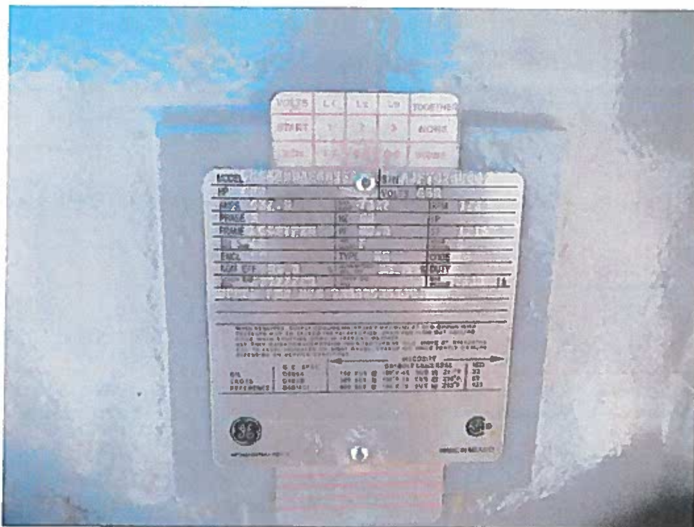
Photo 4 – Motor Name Plate for New Well 2
