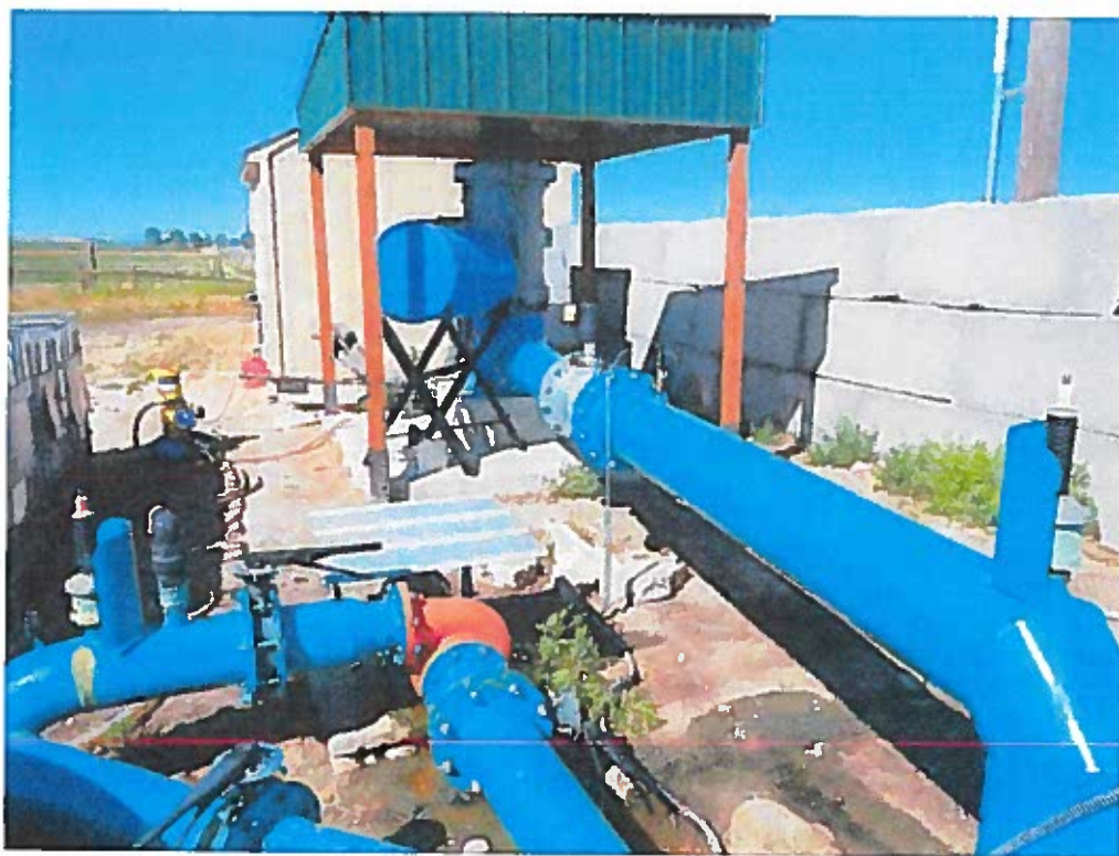
Photo 5 - 7½ HP Booster at the New Well 2 Location
