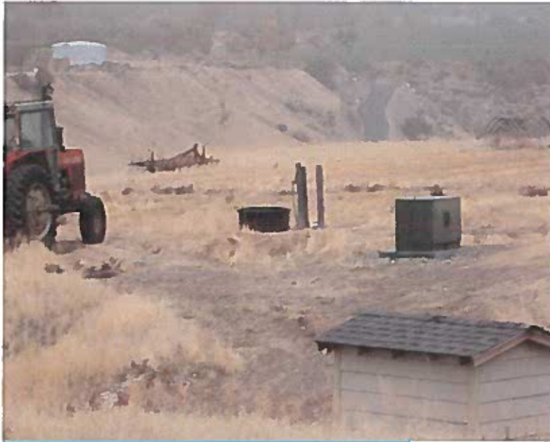
7 frost free hydrants on 7 empty lots
