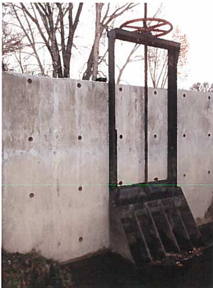
Below: The top of the 24" culvert with headgate in place.
