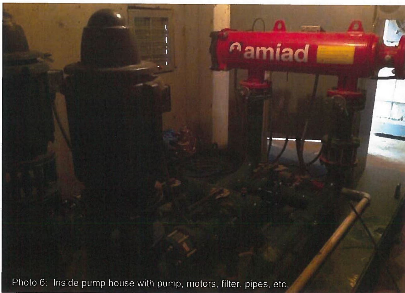
Photo 5: Inside pump house with pump, motors, filter, pipes, etc.
