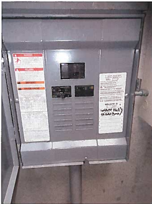
Electrical box inside well house
