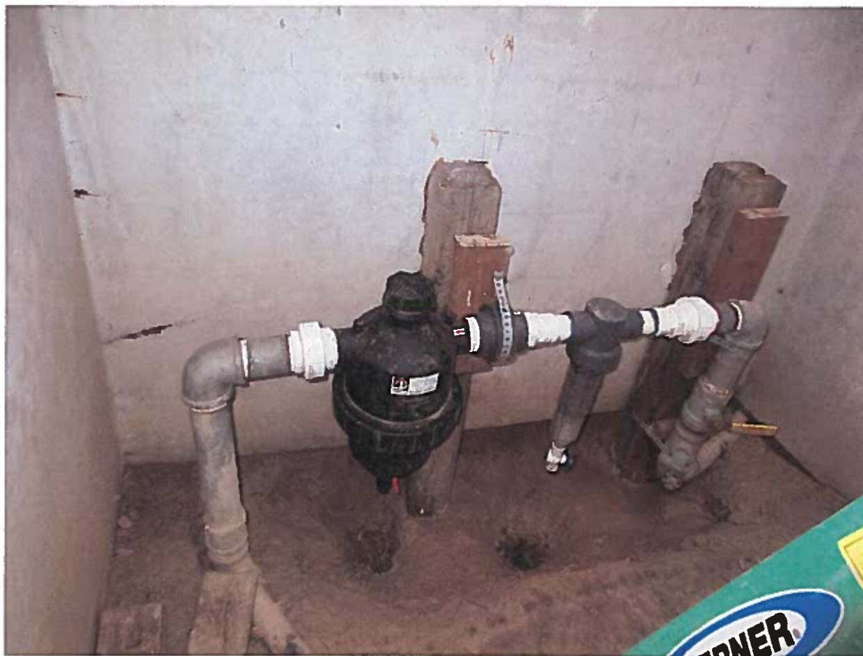
Pipes inside the well house
