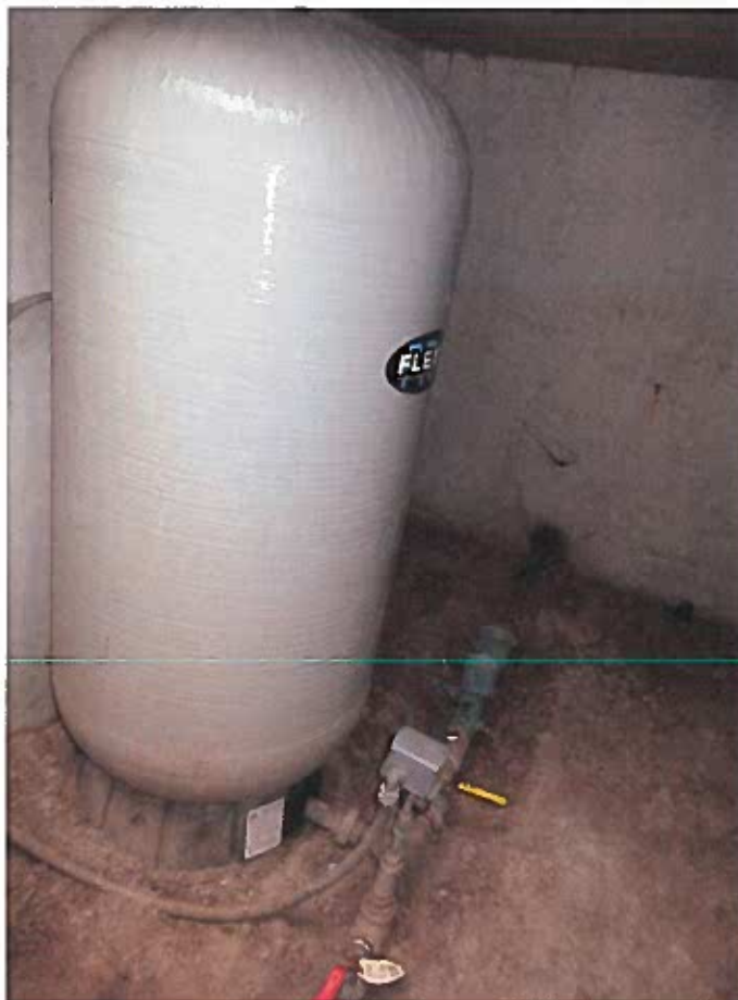
Looking at the pressure tank inside the well house
