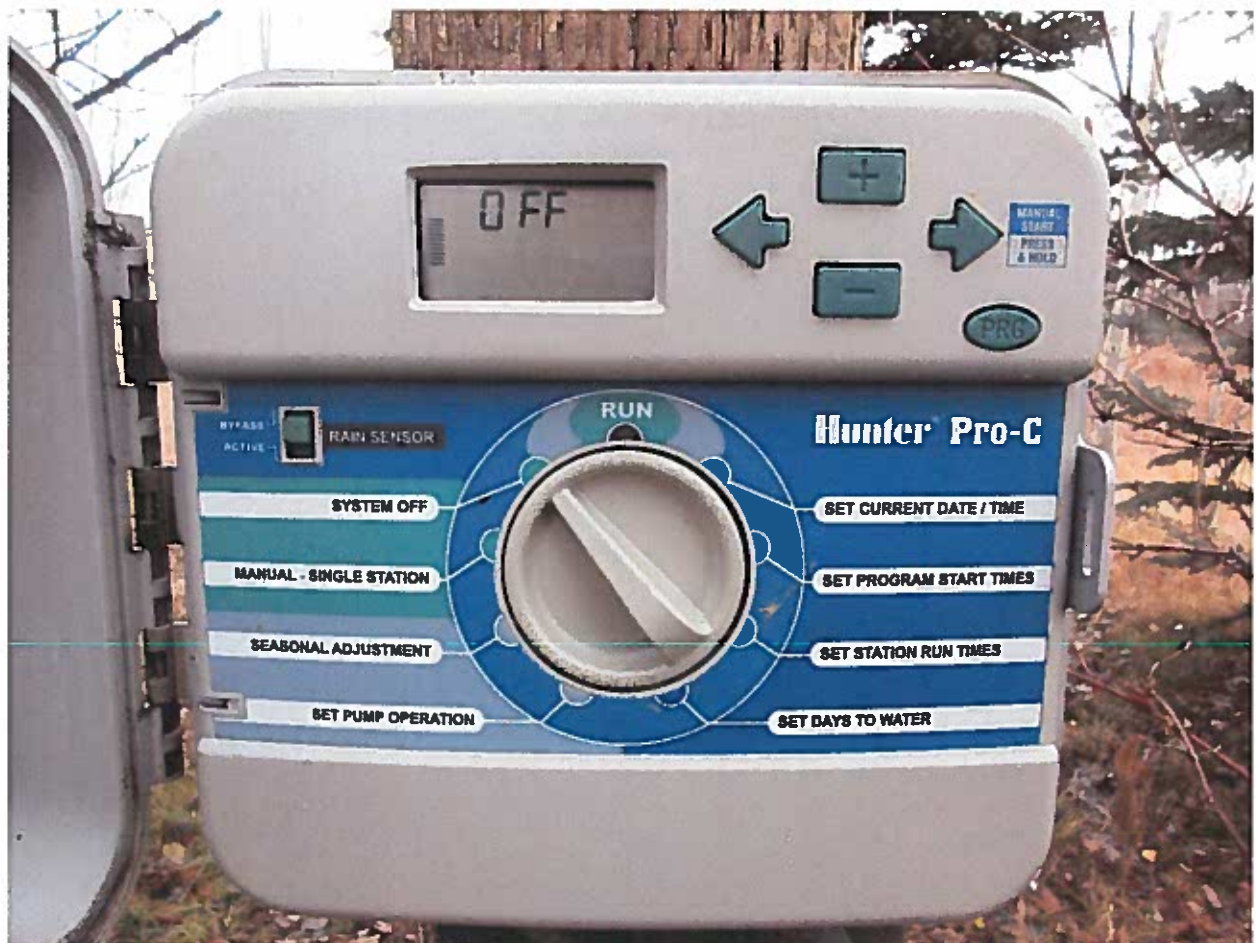
Control box next to pond
