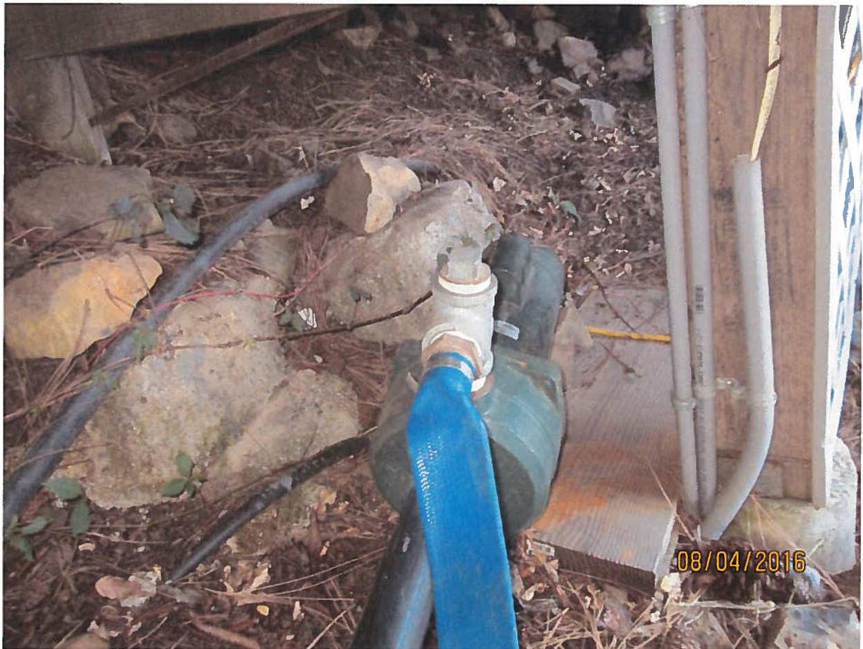
Water intake line on bottom to pump and fire protection hose in blue.
