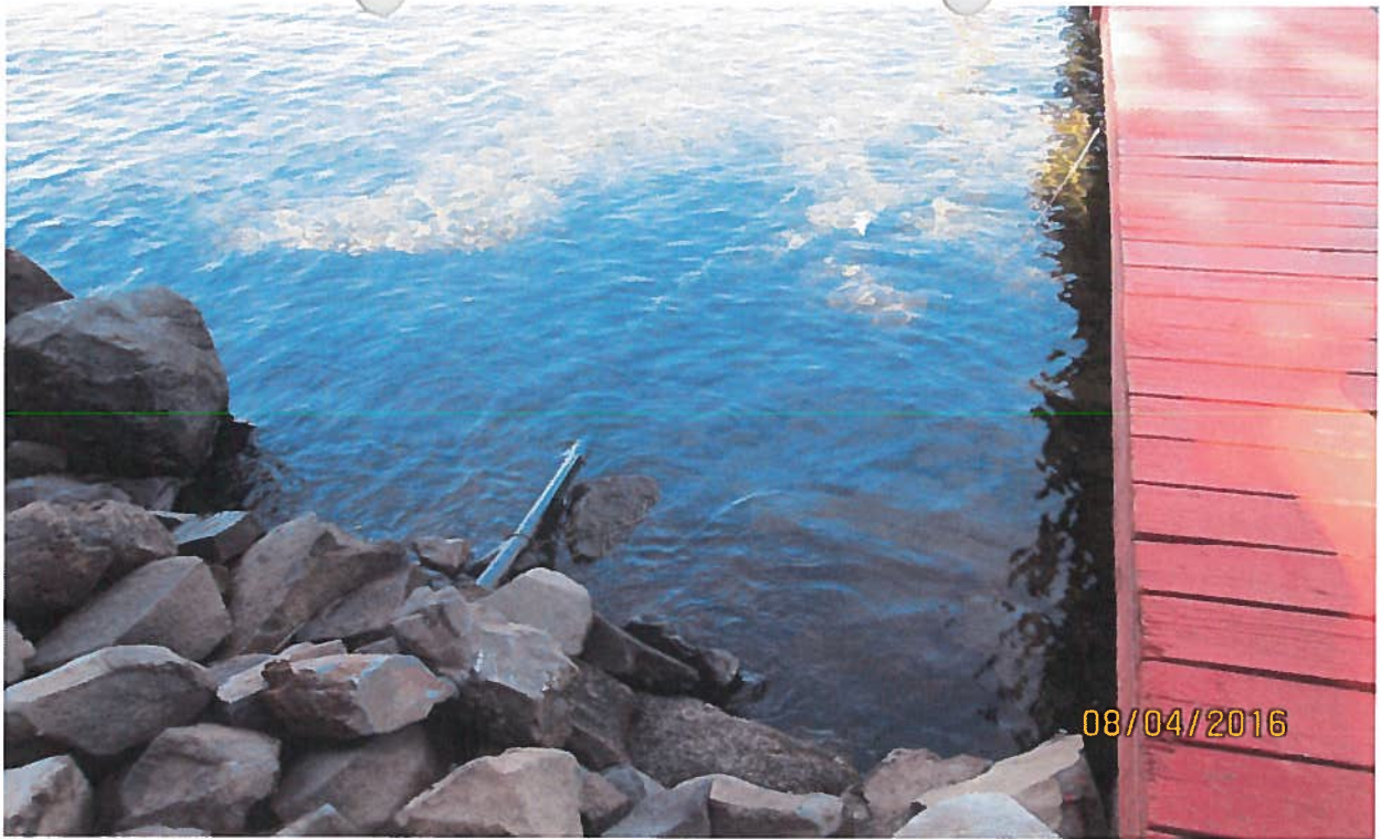
Pipe from lake to pump.
