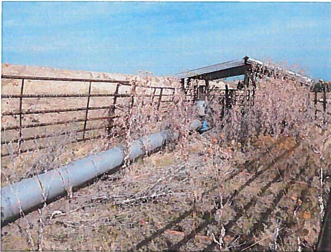
67-14250 Site Visit 9/23/2014: POD "Diesel Pump" well (D0029055).
