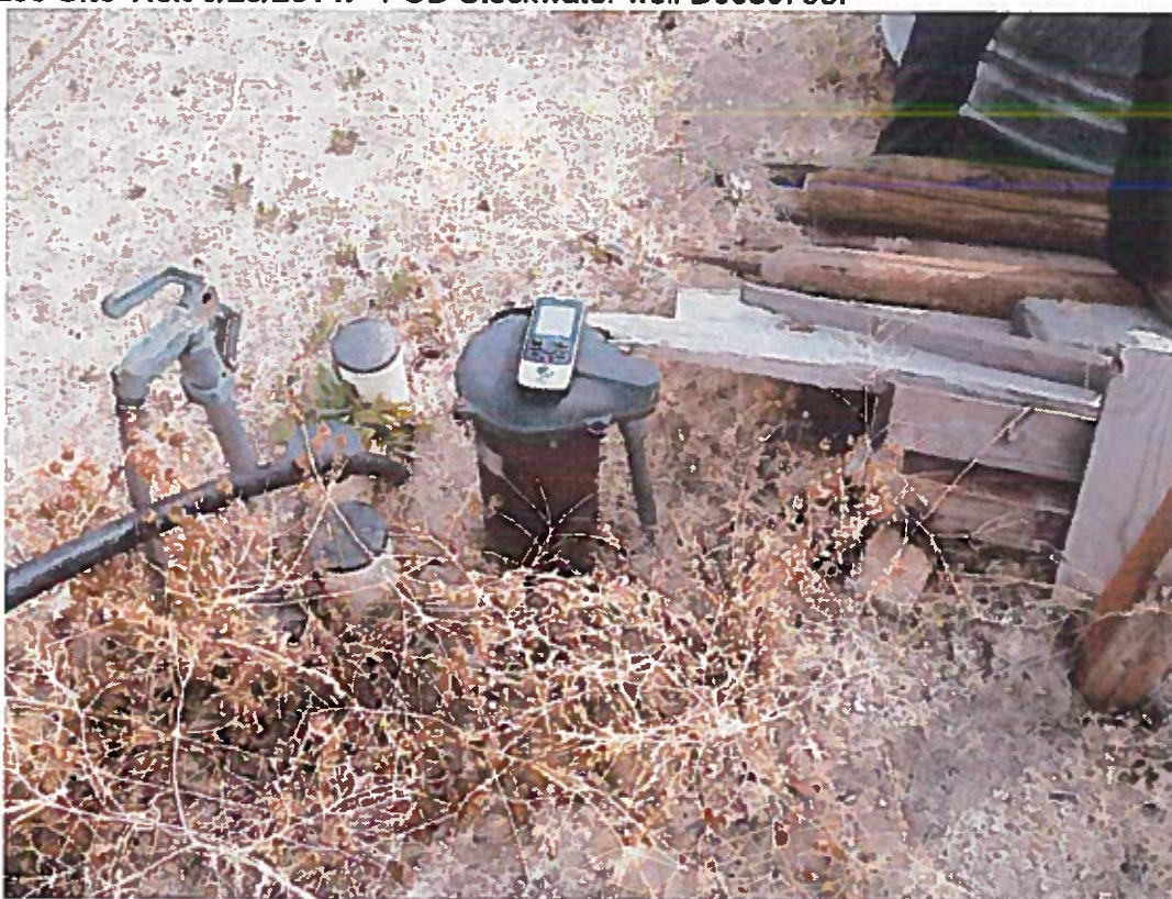
67-14250 Site Visit 9/23/2014: POD Stockwater well D0025990.
