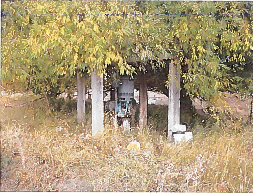
67-14250 Site Visit 9/23/2014: POD "Big Pump" well (D0015099).
