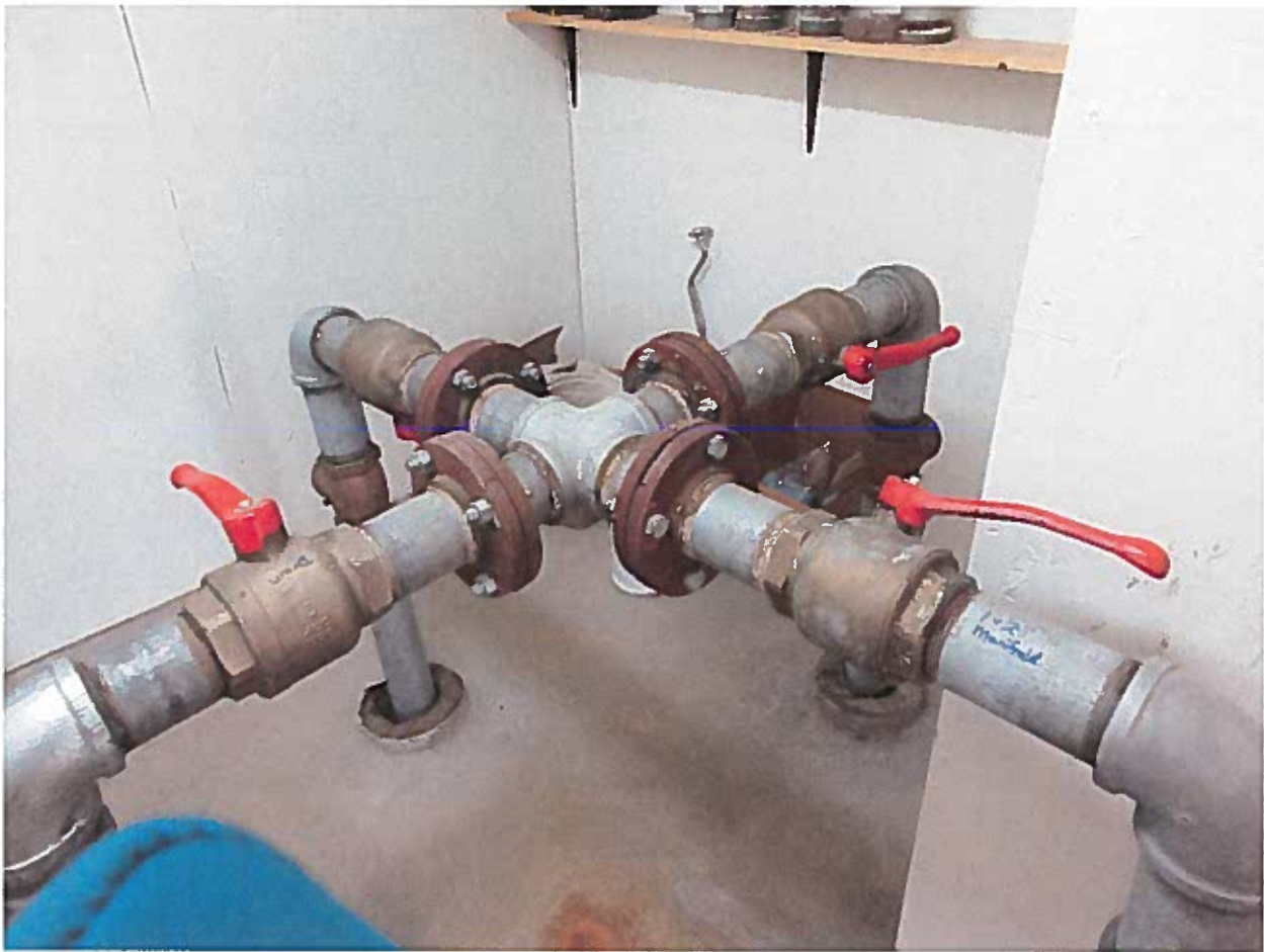
Looking at the pipes routed in the pump house for well 1 and 2
