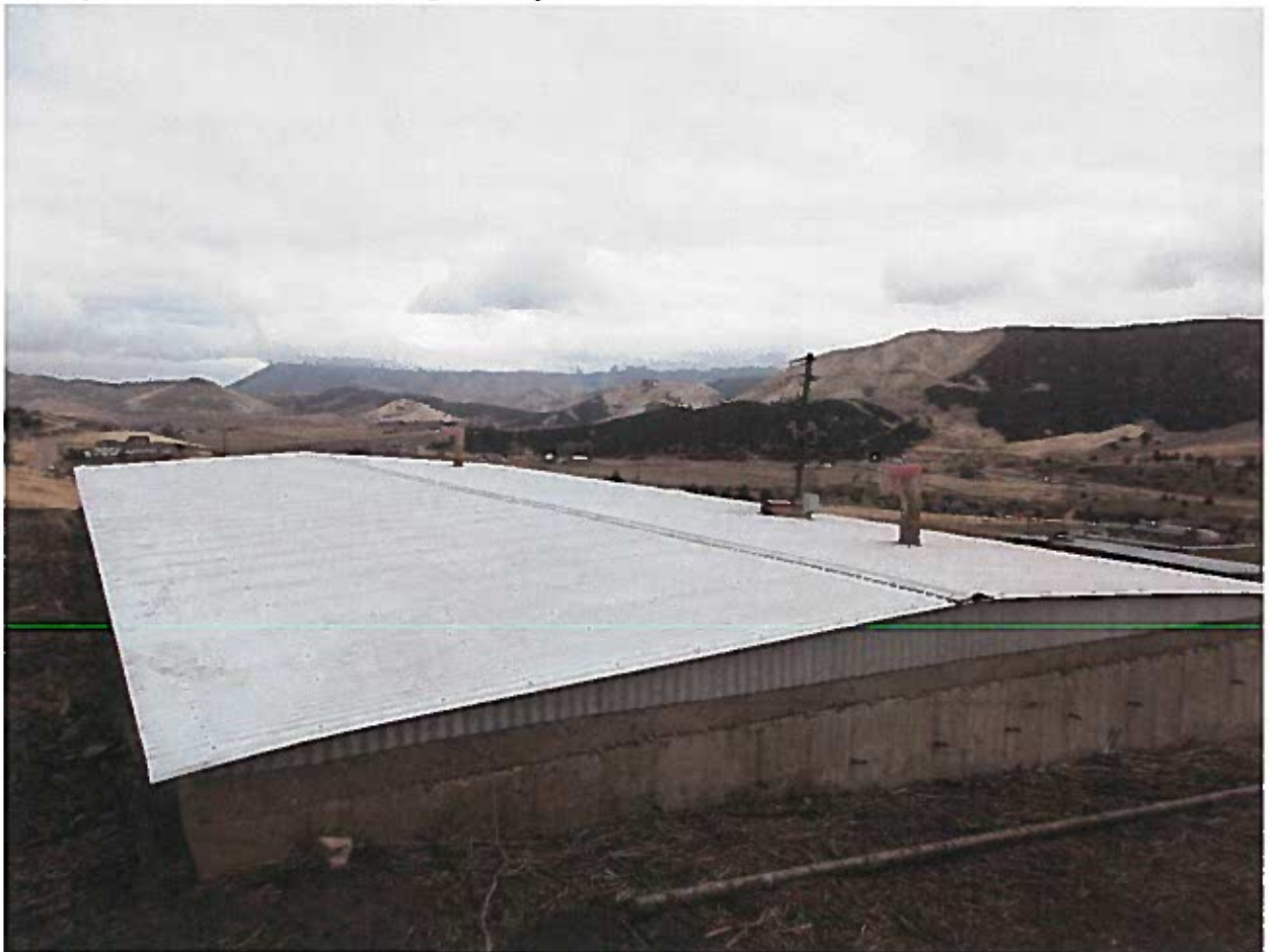
Looking north east at the ~100,000 gal storage tank
