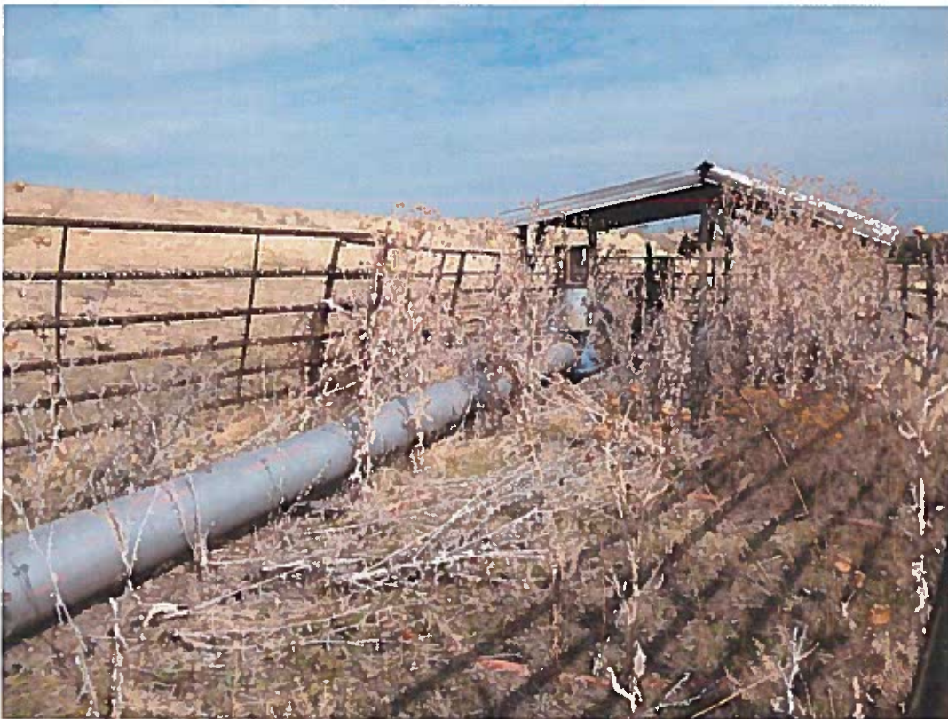
67-14250 Site Visit 9/23/2014: POD "Diesel Pump" well (D0029055).
