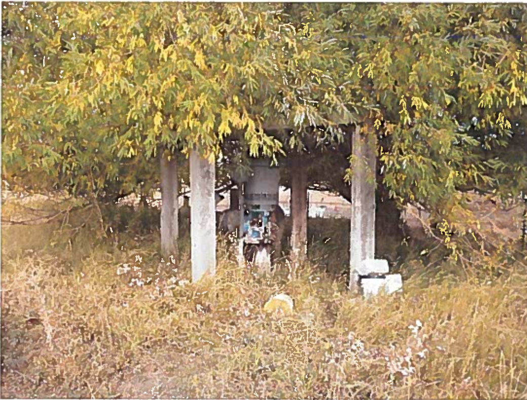
67-14250 Site Visit 9/23/2014: POD "Big Pump" well (D0015099).
