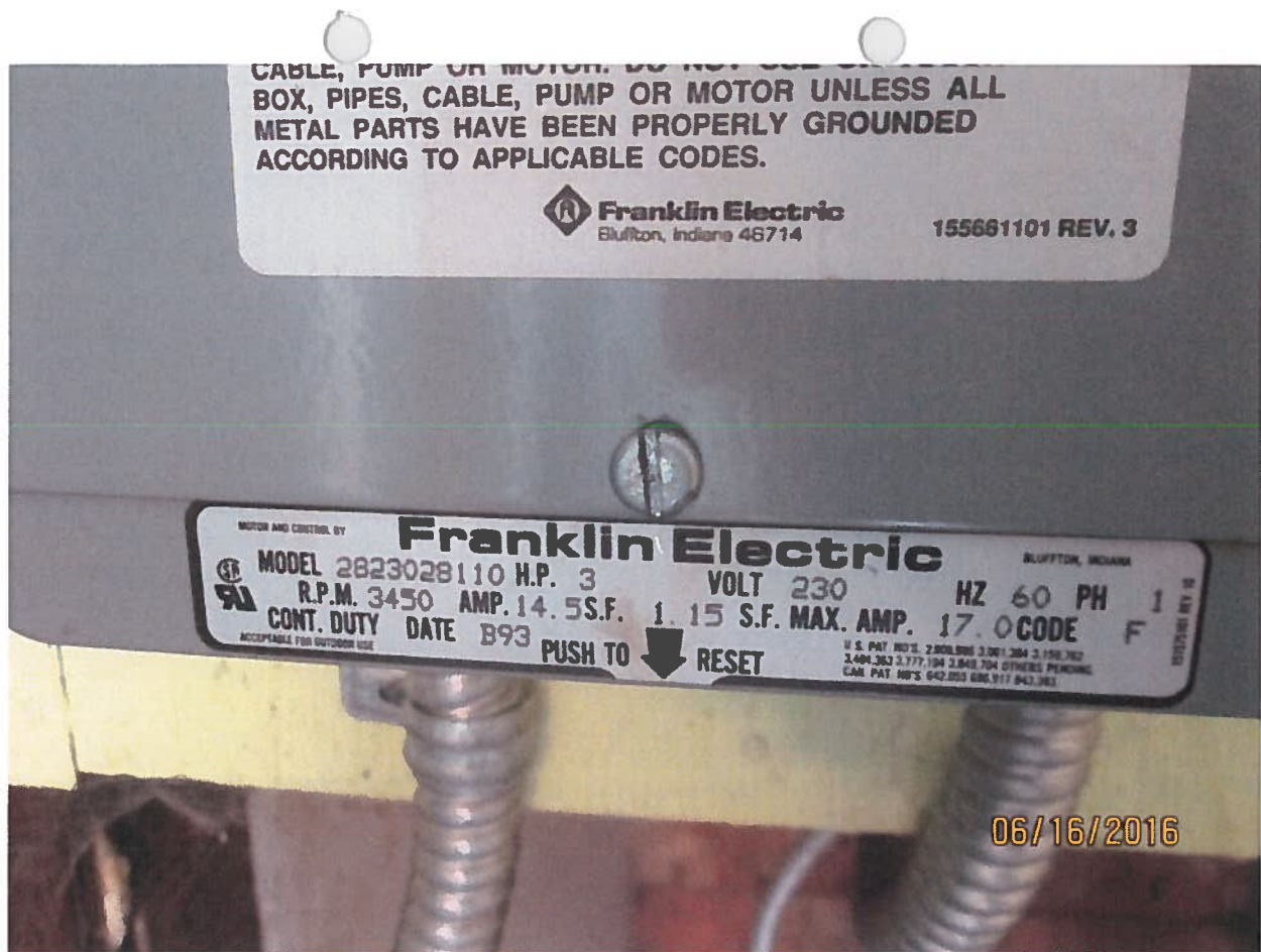
3 hp pump in well.
