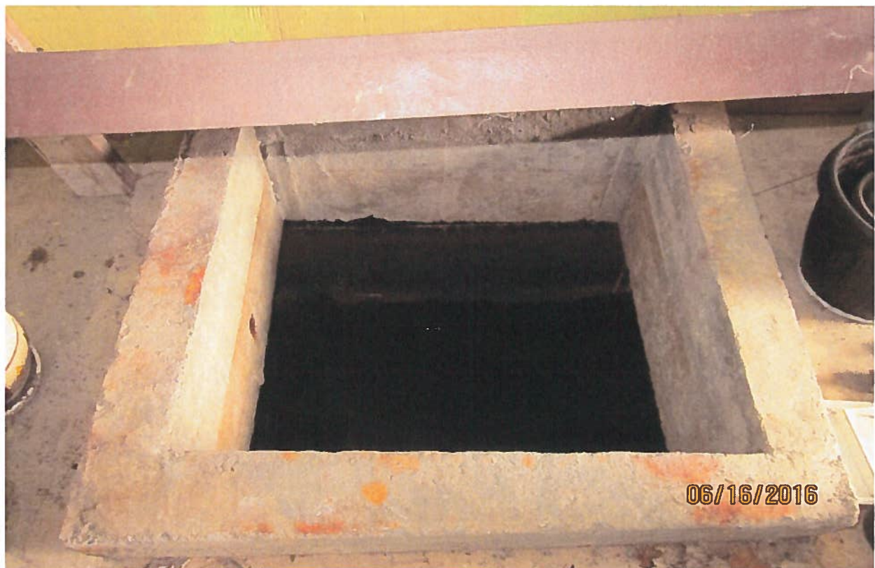
Well pumped in small storage tank under pump house before it was pumped to irrigation and home.
