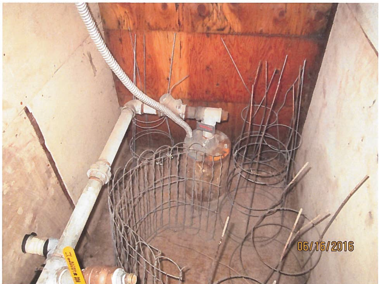
Well drilled in 1976. See attached theoretical pumping equation; estimates flow rate at 23.6 gpm or 0.05 cfs.
