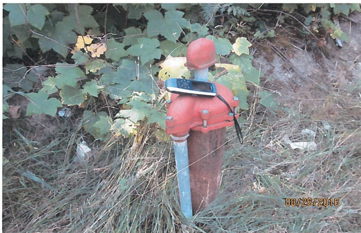
WELL AT BOTTOM OF THE HILL BELOW HOMES. WELL WAS DRILLED IN 1979 TO A DEPTH OF 195FT. UNABLE TO CONFIRM HORSE POWER PUMP BECAUSE LOCK HAD BEEN CHANGED ON PUMP HOUSE. AL VOKING SAID HE INSTALLED AN 18 GPM 1.5 HP PUMP IN WELL.
