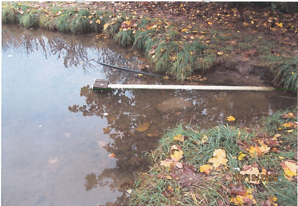
Piping from pond for irrigation.
