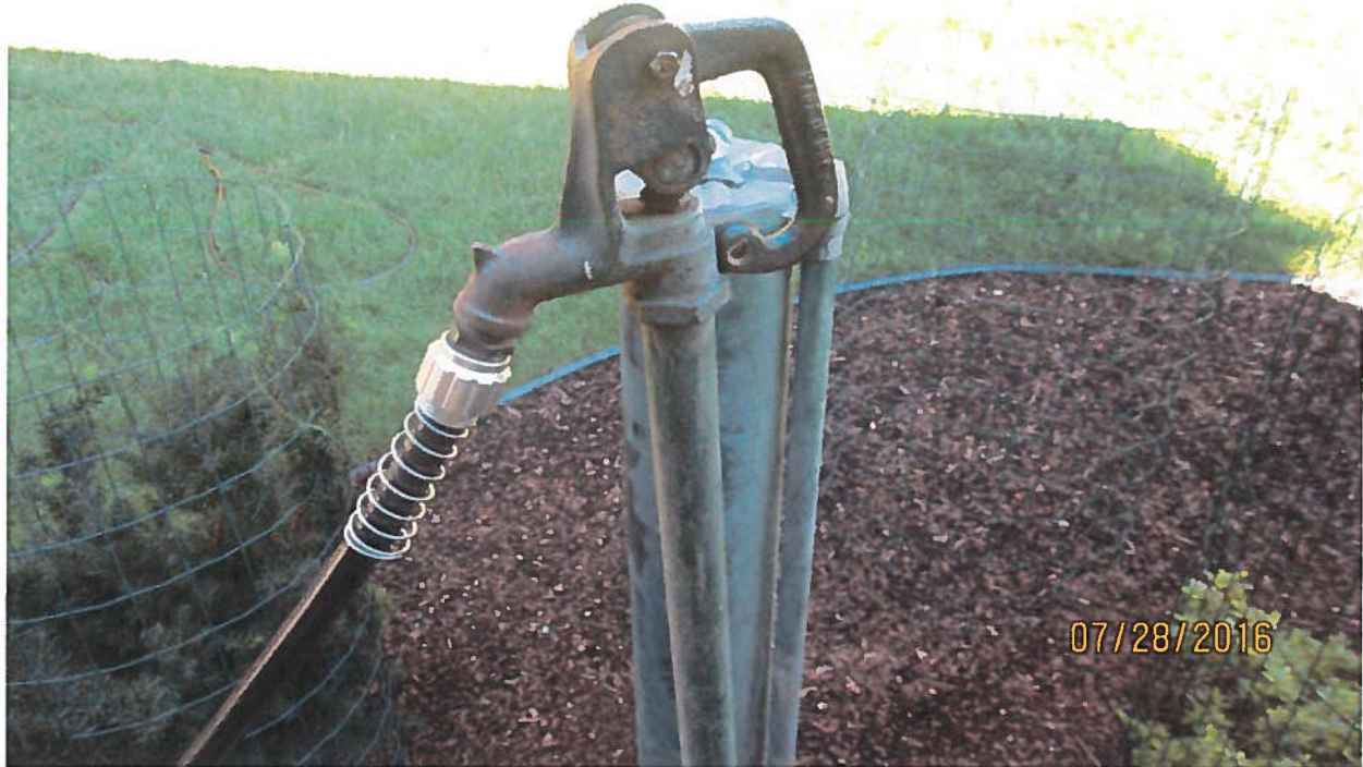
Frost free hydrant where 5 gallon bucket test was performed in 9 seconds.
